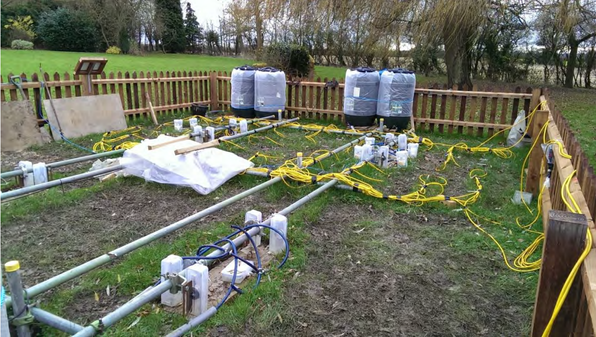
Figure G-23: Completed setup
