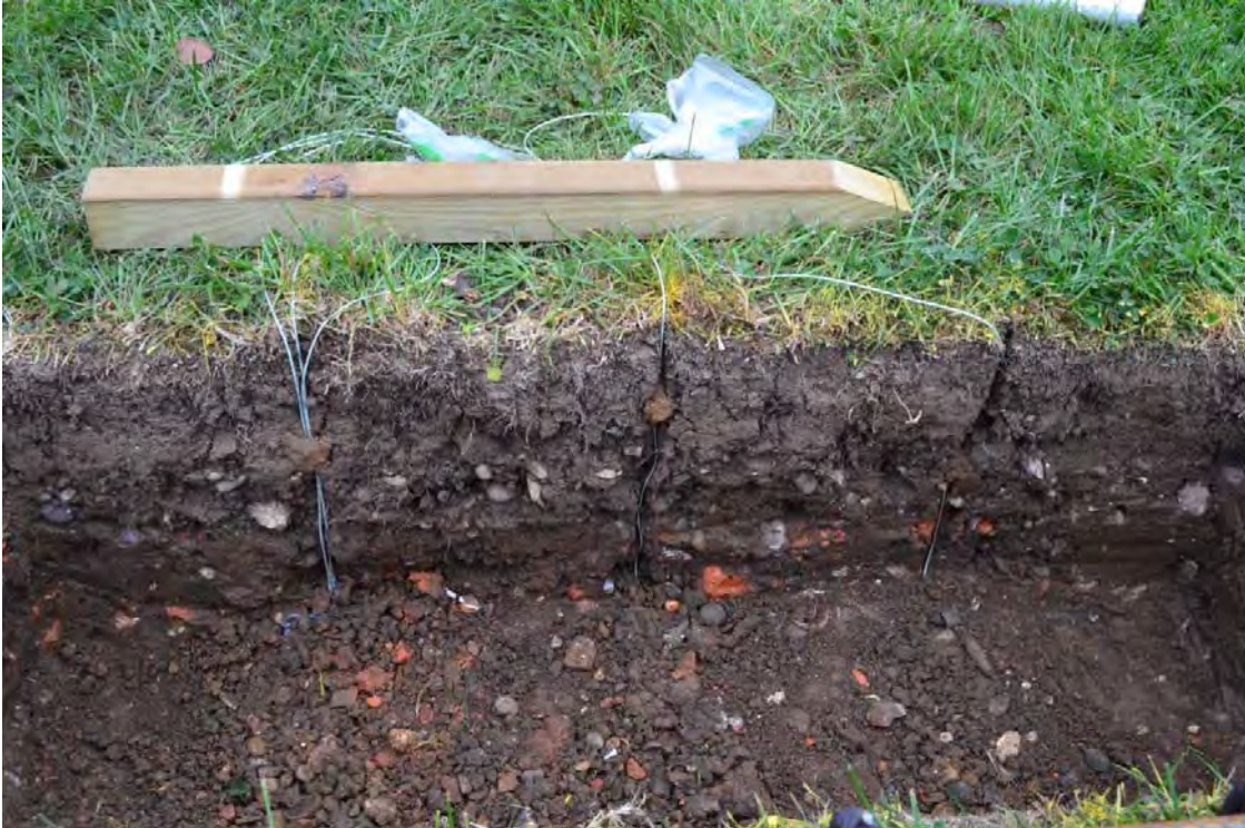
Figure 5-13: Thermocouples buried under clay with wiring hidden in channels in the side and base of footing excavations.
