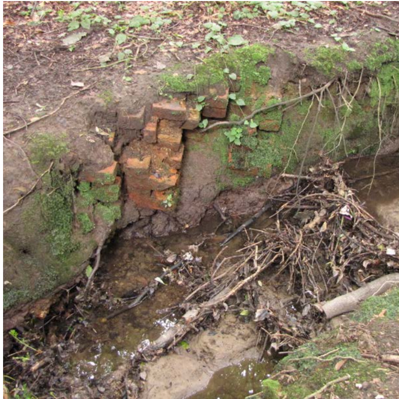
Fig. 7.14: Foundations to the plinth of Maria Dolman's Urn undercut by the present course of the brook. 865
