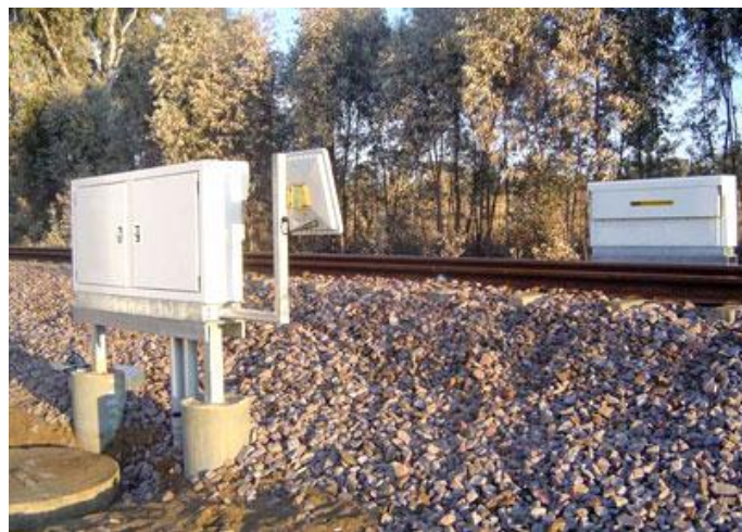
Figure 2.1- Track IQ company hot box detector [37]
