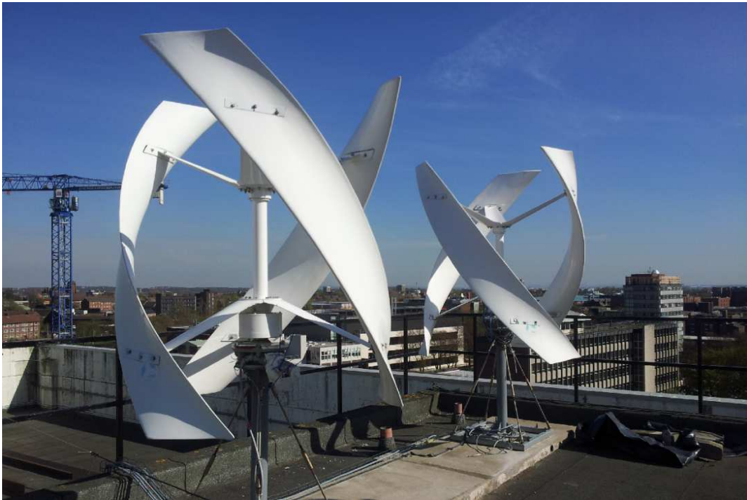
Figure 6.2: The two full-scale vertical-axis wind turbines installed on the building roof of the EEE department
