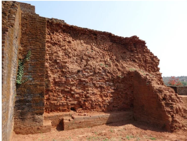
Figure 9-3. Damage caused by rains to the southern side of MNS II. Inner courses of brick have been revealed across this structure and at MNS III.
