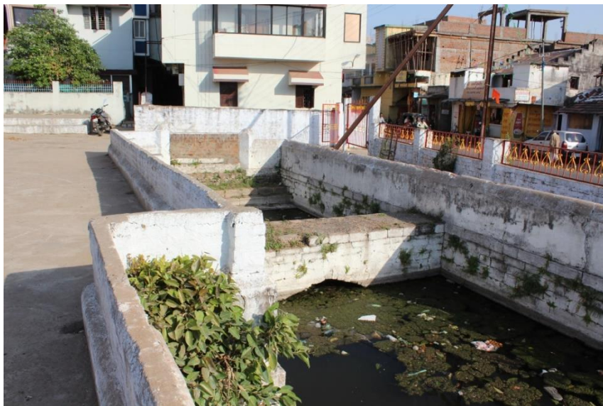
Figure 8-16. The bāvlī in a temple complex in Rāmṭek town (site 119), which has since been filled in and concreted over.
