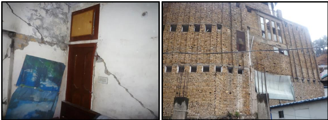
Figure 7.7 A damaged house in Bagh city which has been partially repaired and still inhabited by the owner and his family (left). A pre-earthquake multi storey commercial building in Bagh city, non-frame structure and cracked walls pose serious threat (right). (Source: Author fieldwork)
