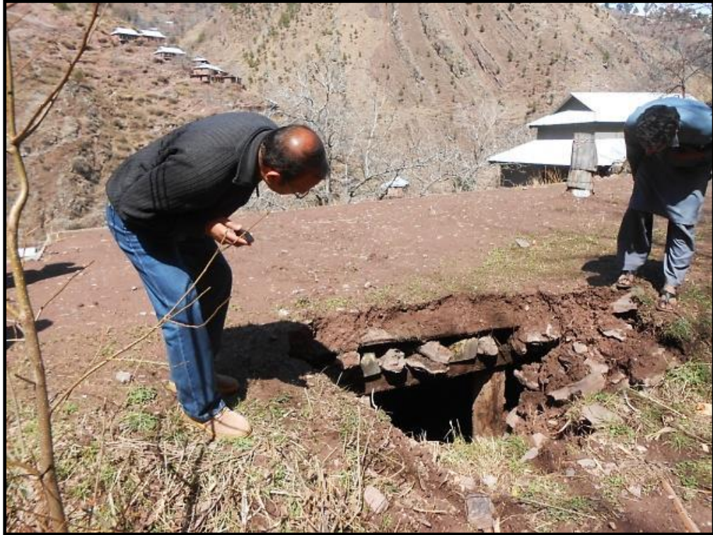
Figure 7.15 Inspecting kacha house damage by a tree which rammed into the wall in village Nalla Katha.
