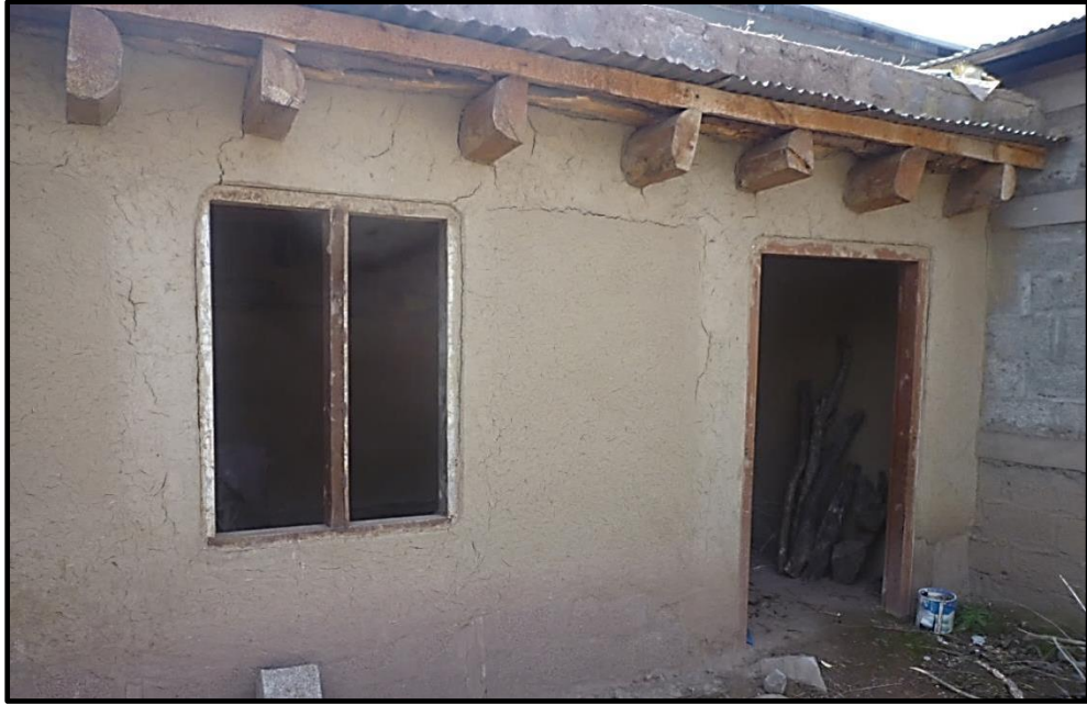
Figure 5.10 kacha (left) and pakka (right) structures side by side in rural Bagh.
