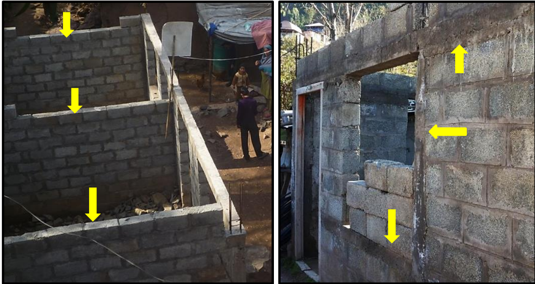
Figure 7.1 (left) An under-construction pukka house in rural Bagh with no plinth and lintel level beams in walls (yellow arrows) in contravention to the ERRA specifications; (right) a seismically compliant under-construction pukka house in rural Muzaffarabad with proper pillars and beams. (Source: Author fieldwork)
