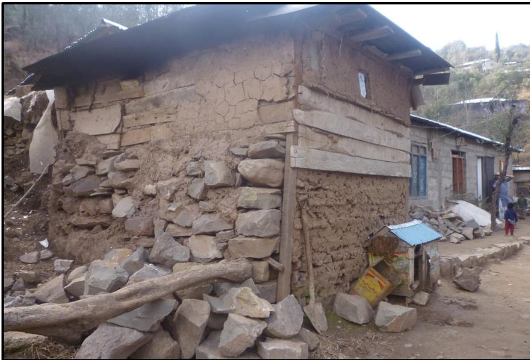
Figure 7.8 A poor quality structure (foreground) added with a reconstructed house (background) in Bagh city; notice different types of materials and irregular stones used in the added structure. (Source: Author fieldwork)
