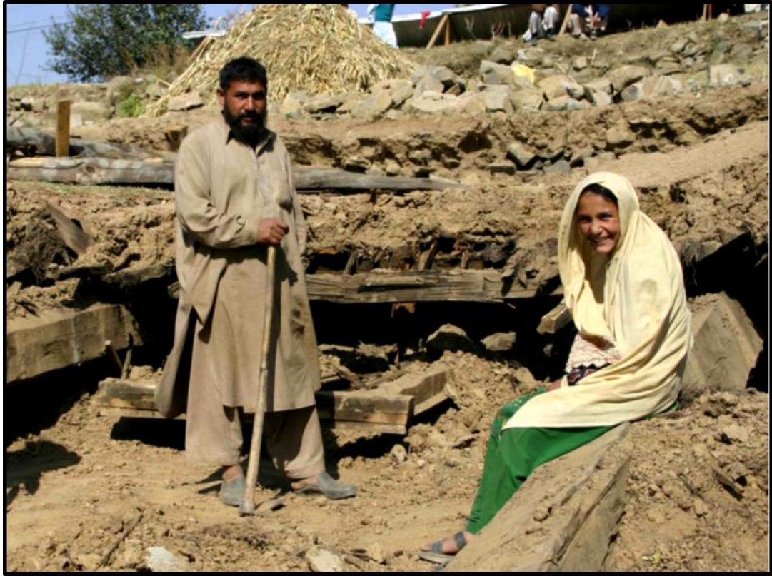
Figure 5.8 A destroyed Kacha house: note heavy wooden beams, loose joints, undressed stones and thick mud roof. (Source: ERRRA 2015)
