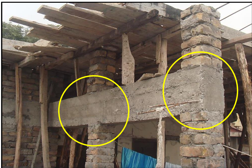
Figure 7.2 An under-construction house in Muzaffarabad city; notice brick columns and concrete beam in utter violation of the engineering principles (yellow circles). (Courtesy: Sheikh Ahsan)
