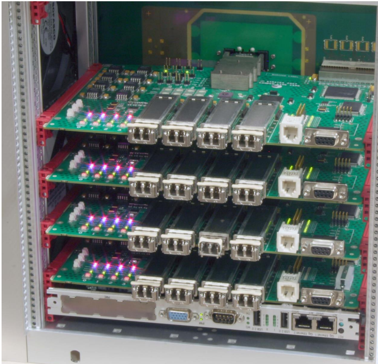
Figure 4-49: FirstLight demonstration platform fully populated with all four test line cards and powered up
