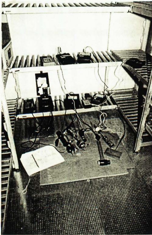
Figure 3-1: Resistance-type moisture meters in the walk-in freezer environment (-10 °C temperature)
