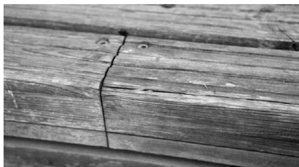
Figure 7 Rounding of edges and break ups of TMT-gluelam in service
