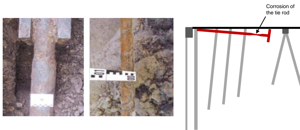
Figure 12. Photos of tie rod corrosion at a quay wall in a harbour of north Germany (left) and principle sketch of the location of the corrosion (right).
