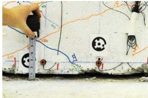
(b) Wall 8 web separation
