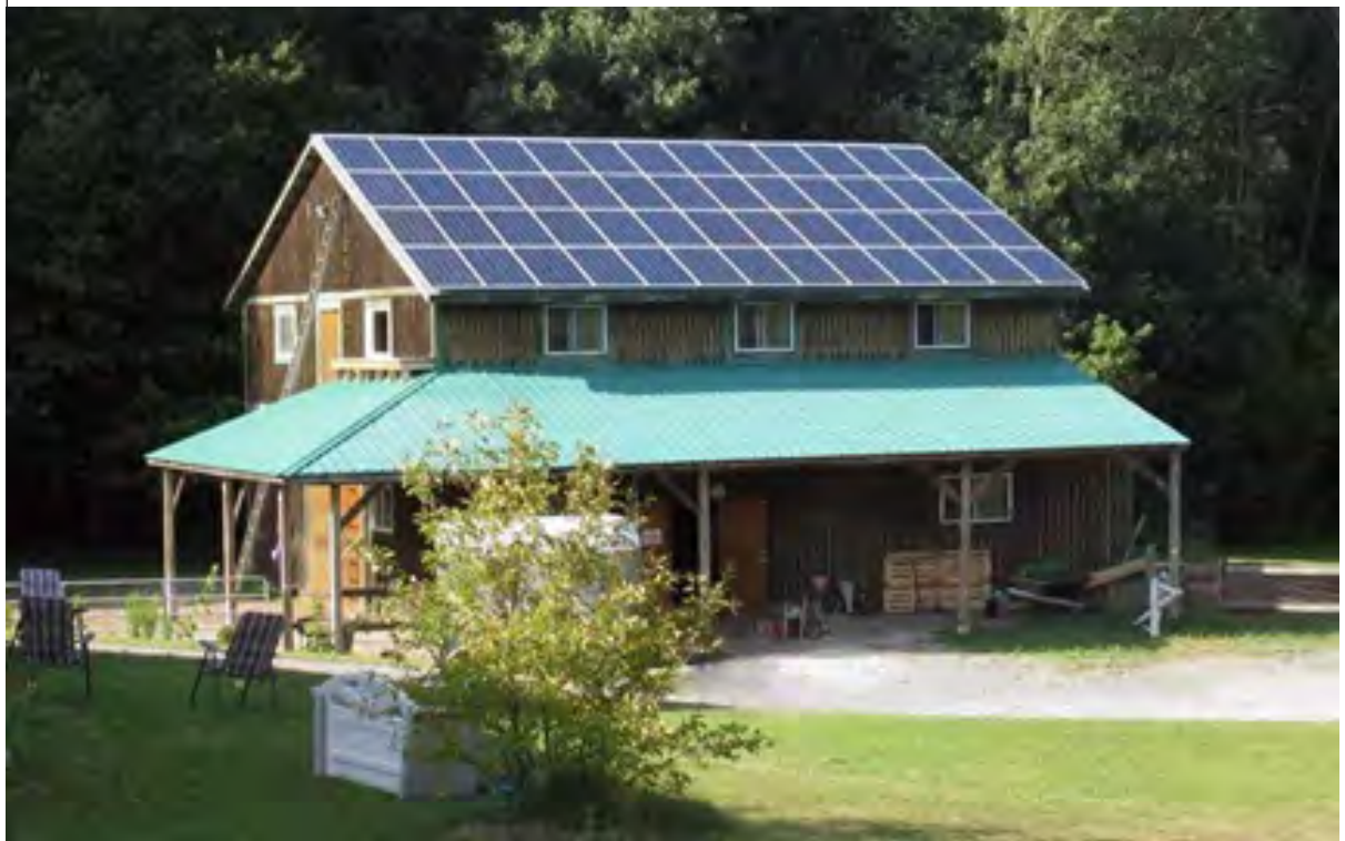
Figure 5-12: Residential solar panels
