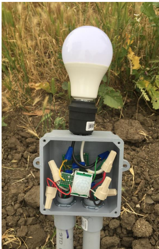
Figure 5-2: Junction box to house circuitry
