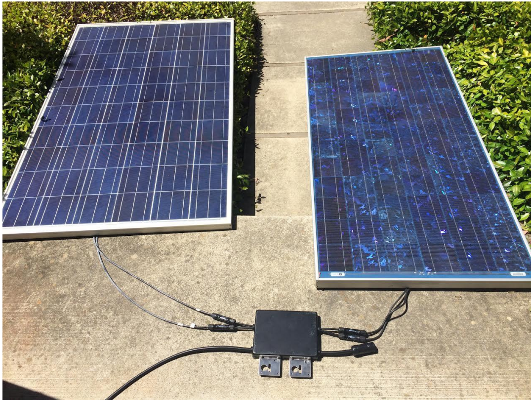
Figure 5 - 1: Solar panels connected to microinverter with MC4 plugs
