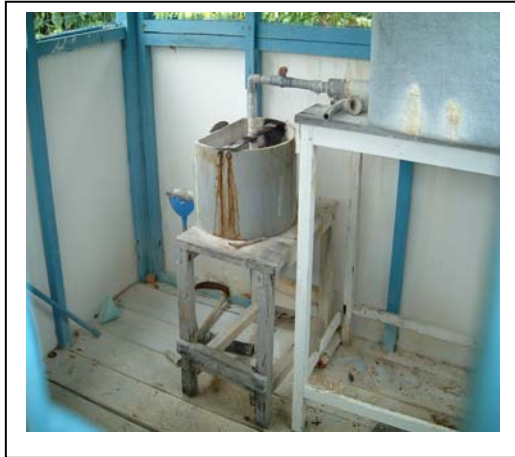
Figure 12(c) – The conventional chlorine dosing tank used by Water Supply Authority
