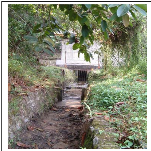
Figure 8(b) – Discharge point of tailrace from the turbine house
