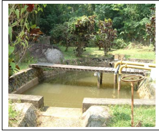
Figure 3 (c) – The water storage in the pump sump
