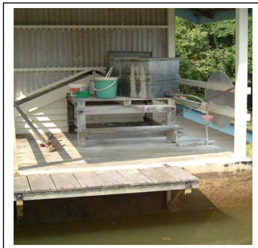
Figure 3 (e) – The chlorination system
