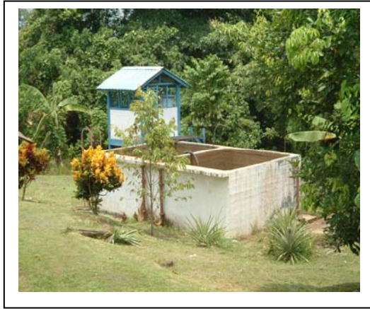
Figure 12(b) – The slow sand filter water treatment plant and chlorinator housing
