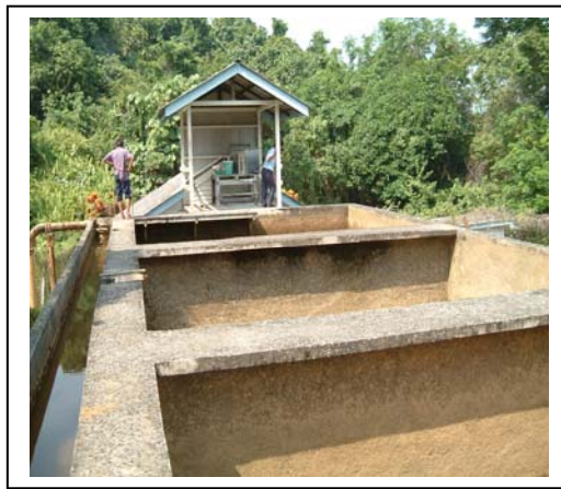
Figure 3 (d) – The slow sand filter treatment plant
