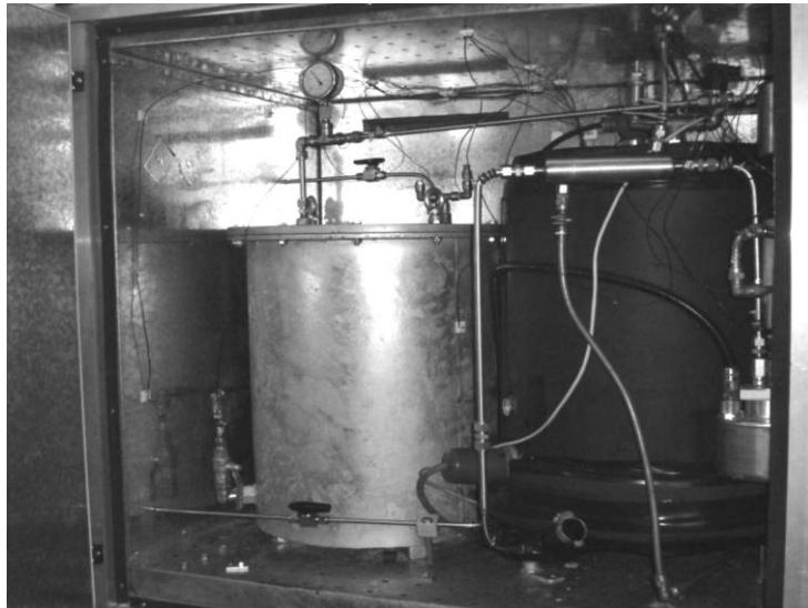
Figure 3: Heat exchangers cabin
