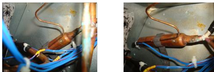
Figure 6: Filter dryer in original (left) and horizontal (right) positions
