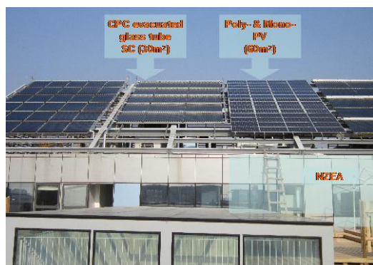
Figure 6: Photo of solar collector array and PV
