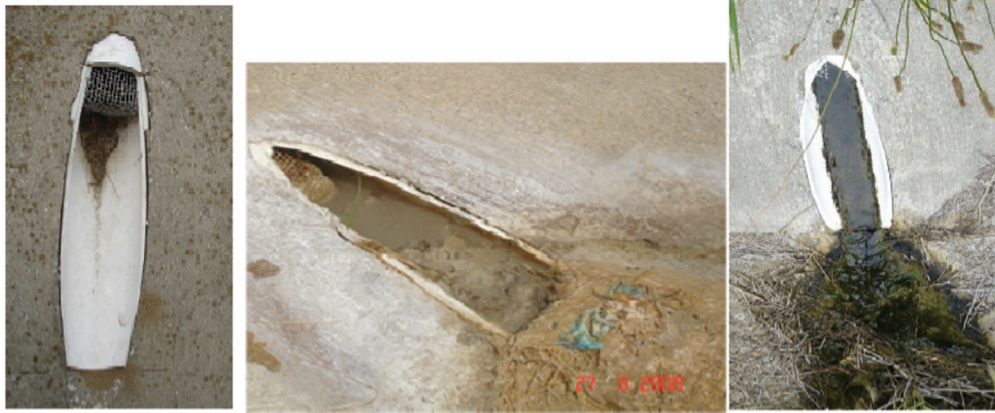
Figure 4.5 The condition of the drain outlets varied.
