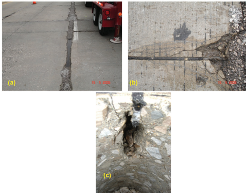
Figure 1.1 Condition of the EB pavement at W. 86 th St. (east of the intersection with N. Payne Rd. in Indianapolis, Indiana, referred to as AL location): (a) general view, (b) close-up of damaged region near the intersection of transverse and longitudinal joints and (c) example of bulb-shaped damage zone under the joint sealant (1).
