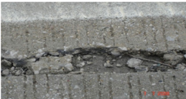
Figure 1.1 Deteriorated longitudinal joint, I-94.
