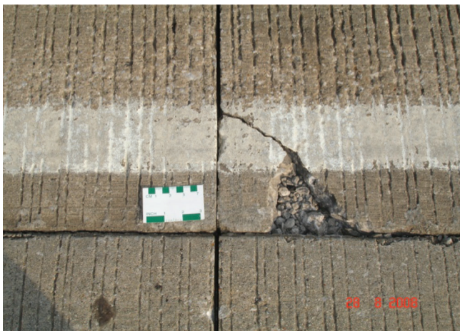
Figure 1.5 Occasional corner cracking in the EB lanes of eastern most portion of this project in the area with unsealed joints (identified as Section 5).
