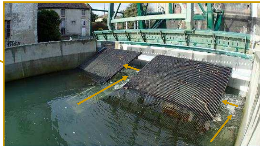
low-sloping racks with 2 bypass entrances
