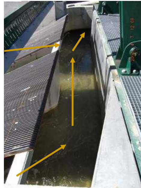
collecting bypass channel
