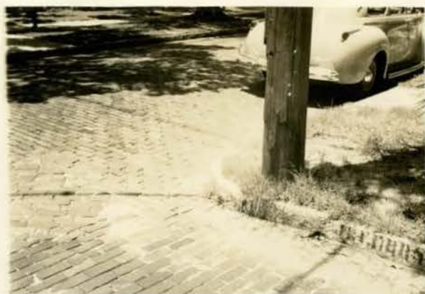
Old type of 3 foot corner curb. These were fine for horses and buggies but now should be widened to a radius of at least 25 ft.
