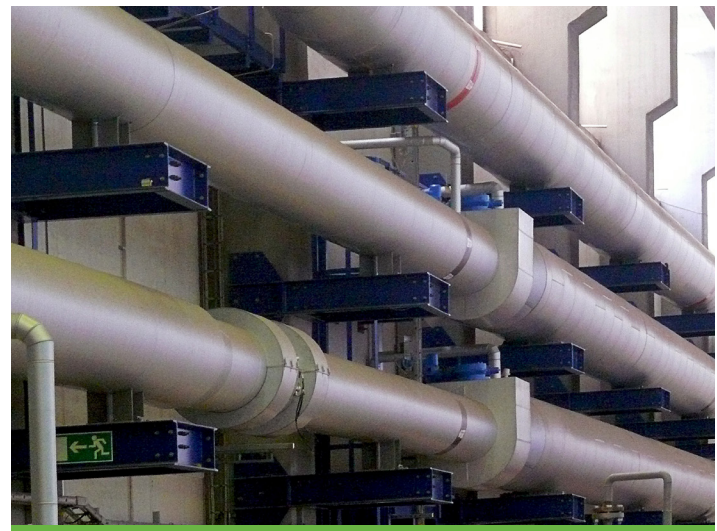
District heating pipes
