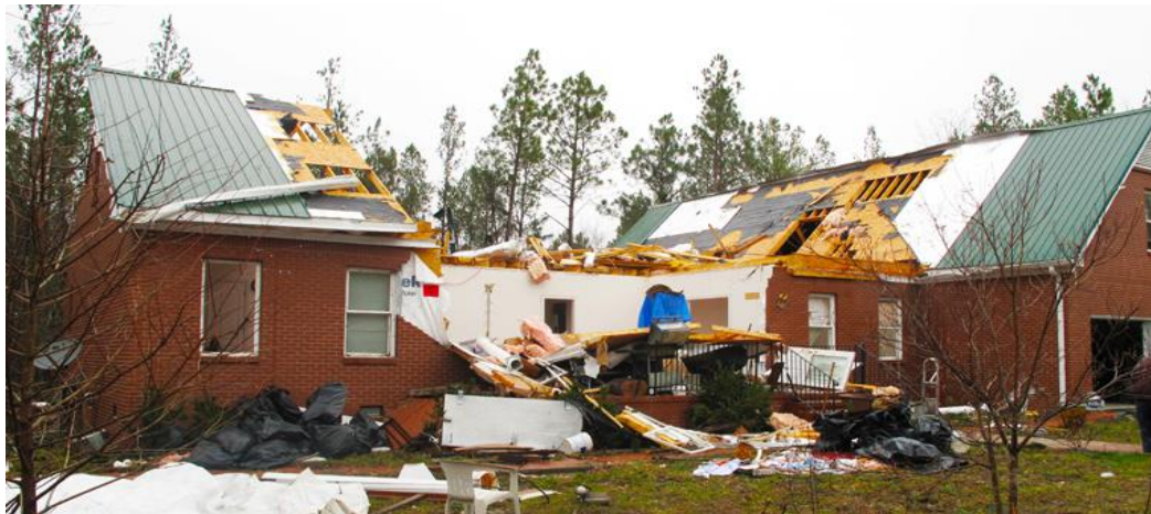
Figure 1.3 RTWC failure and full roof collapse, www.floridadisaster.org
