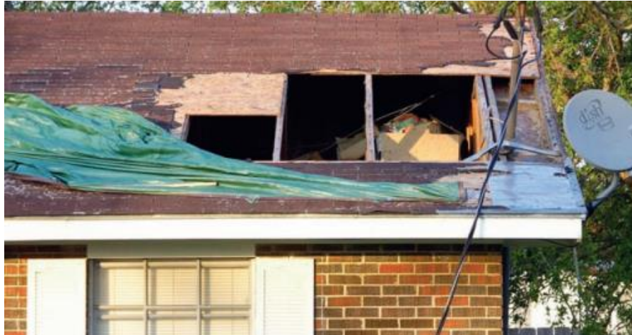
Figure 1.2 STTC failure, www.fema.gov
