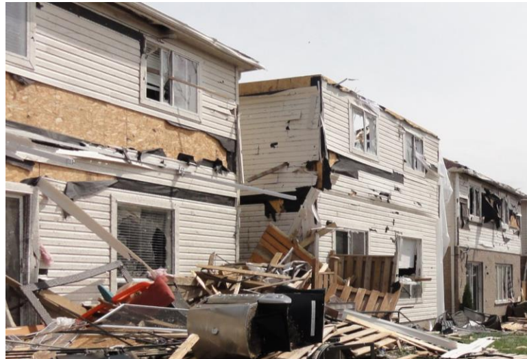
Figure 1-1: (a) Degree of damages (DOD) and the corresponding range of failure wind speeds for typical one- and two-family residences (WSEC, 2006) (b) Examples of DOD 2. (c) Example of DOD 4. (d) Example of DOD 6.
