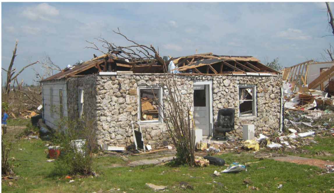
Figure 1-8: Partial hip roof failure in Region 2 (Image provided by Dr. David Prevatt).
