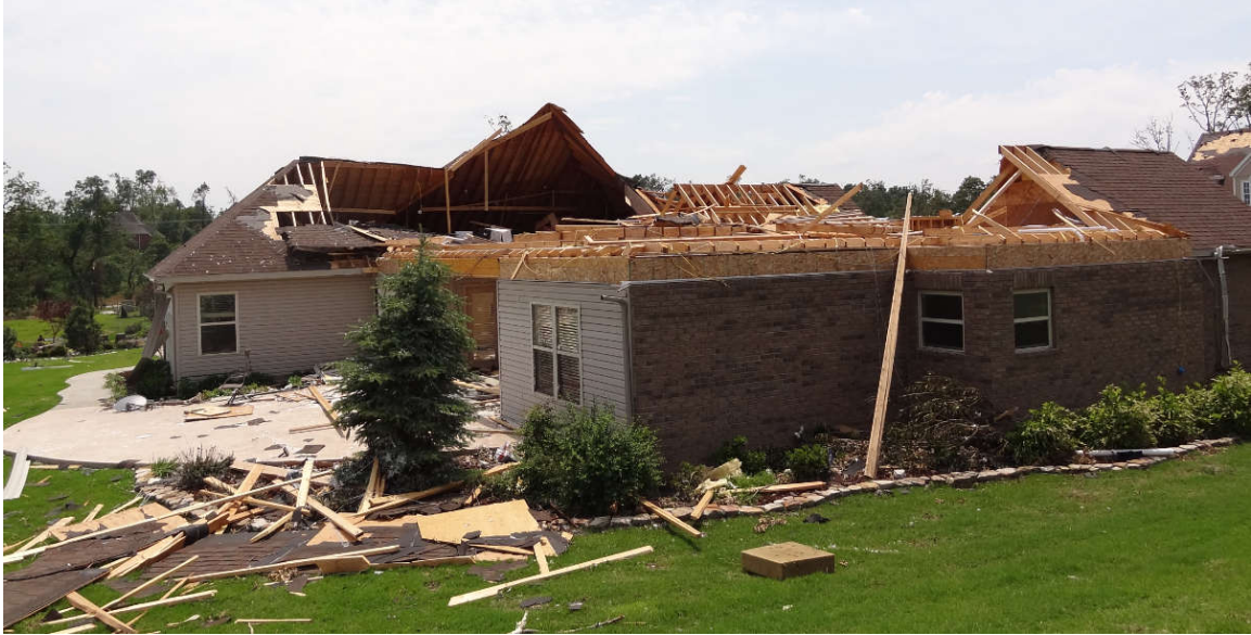
Figure 4-4: Partial stick-frame, hip roof failure with ceiling joists intact (Image provided by Dr. David Prevatt)
