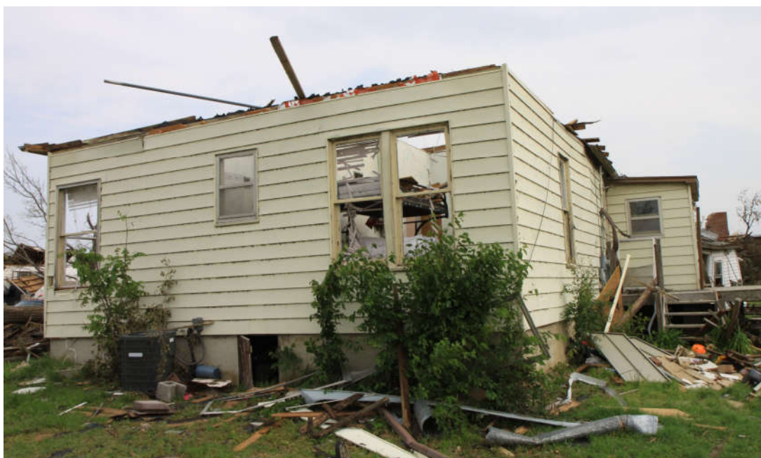
Figure 1-2: Example of roof-to-wall connection failure, corresponding to DOD-6 (Image provided by Dr. David Prevatt)
