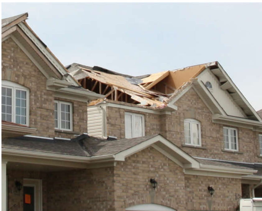
Figure 1-3: Partial hip roof failure observed following EF2 tornado in Angus, Ontario, June 2014. (Image provided by Dr. Greg Kopp)
