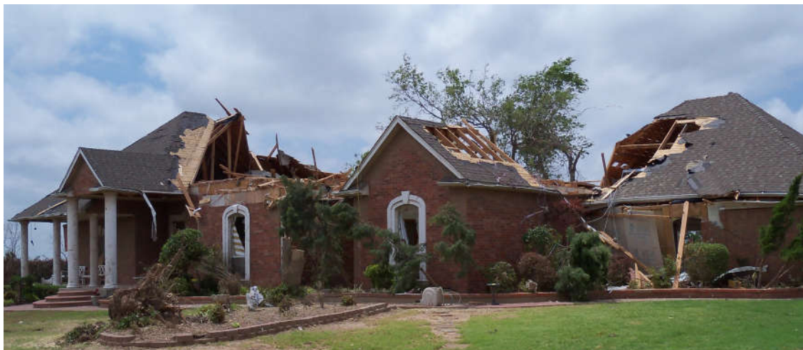
Figure 4-3: Failure of stick-frame roof with irregular roof shapes (Image provided by Dr. David Prevatt)
