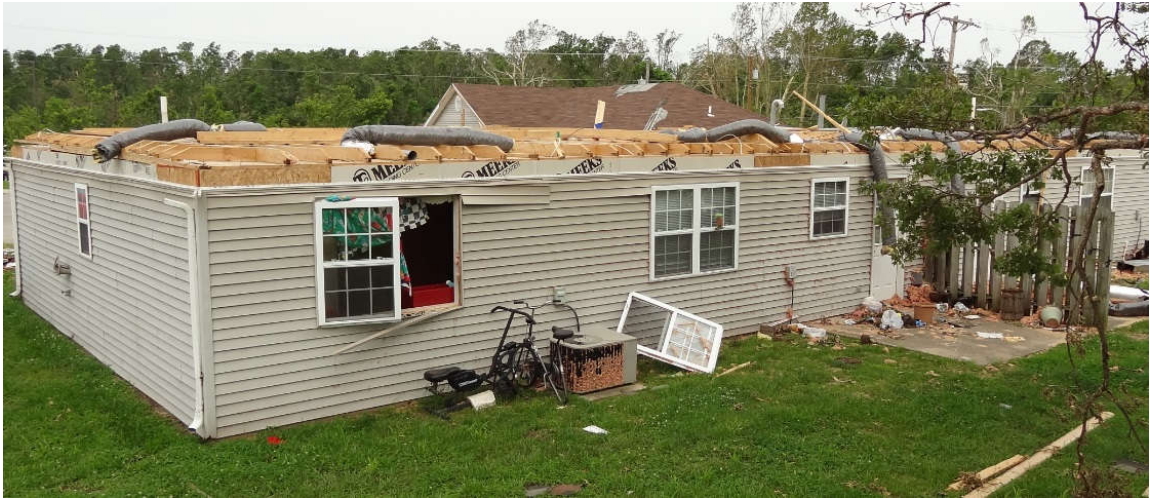
Figure 4-5: Loss of the entire surface of a stick-frame hip roof with intact ceiling joists (Image provided by Dr. David Prevatt)
