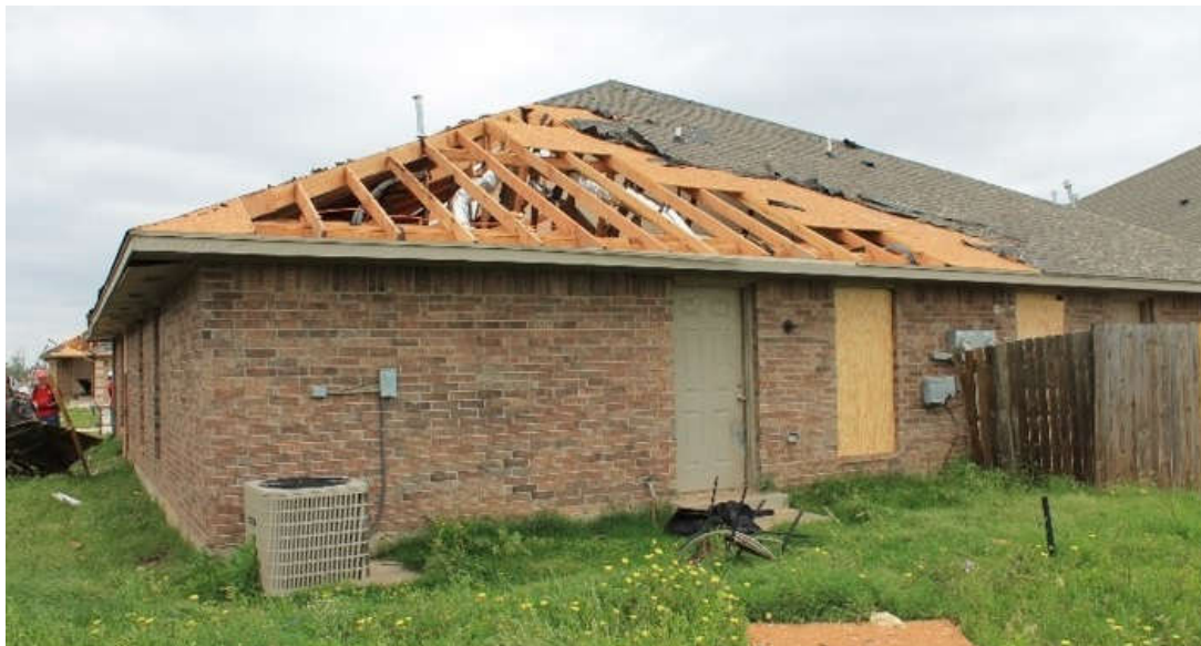
Figure 1-1: Example of roof sheathing failure, corresponding to DOD-4 (Image provided by Dr. David Prevatt of University of Florida)
