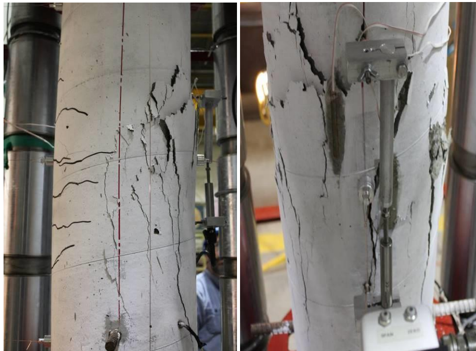
Figure 3: Final crack pattern of specimen C25
