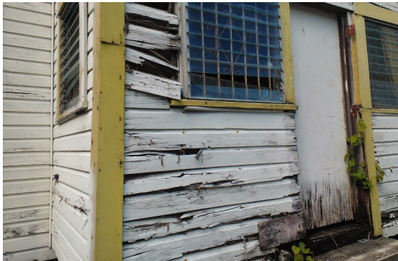
Neglected façade maintenance and upkeep.
