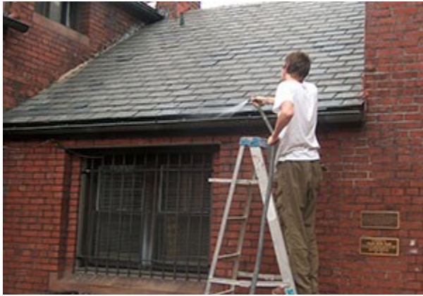
Proper cleaning and maintenance of gutters is essential in minimizing water and debris damage to a historic structure.
