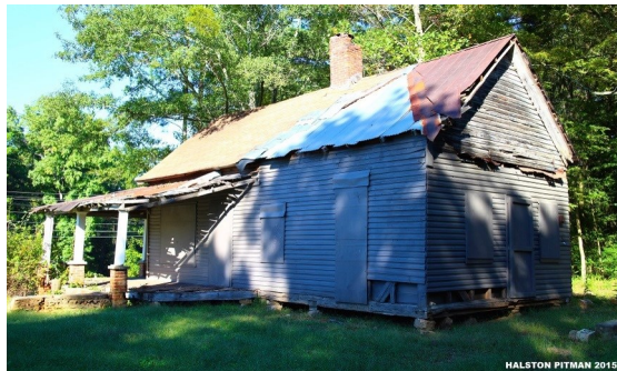
Johns Homestead nominated by Georgia Trust for Historic Preservation's "10 Places in Peril"
