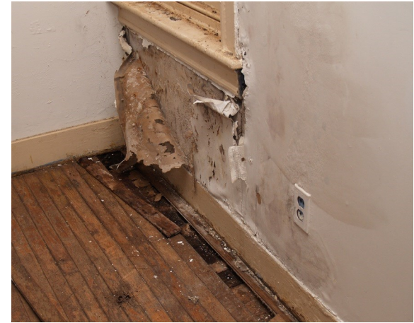
Neglected waterproofing and building maintenance resulting in building foundation issues.
