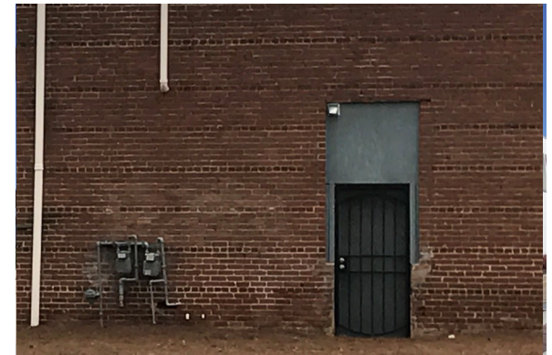
Inappropriate door infill with plywood that ignores the transom.
