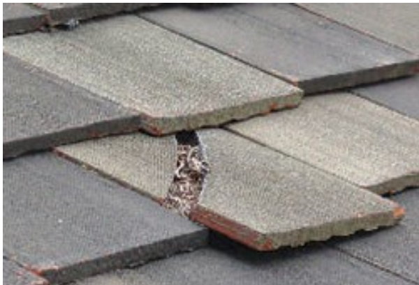
Roof damage and maintenance is vital to address in a timely manner.
