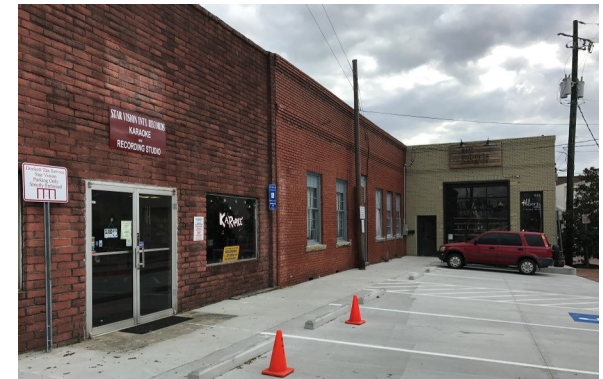
Inappropriate wall sign materials, mounting and scale.
