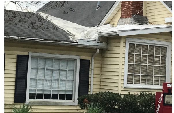
Inappropriate roof preservation with excessive amounts of waterproofing.
