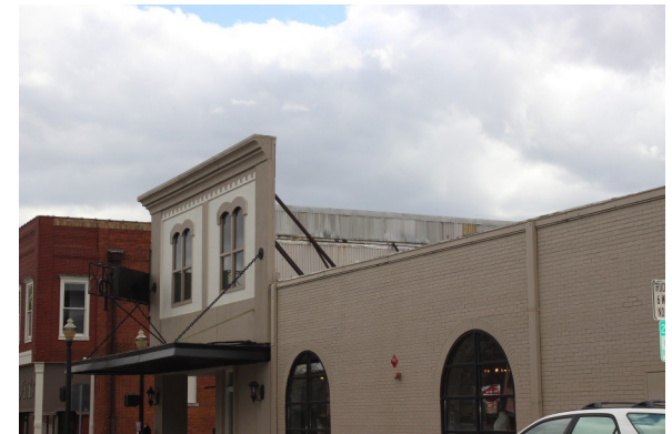
Inappropriate addition to an existing structure increasing the appearance of the building height.
