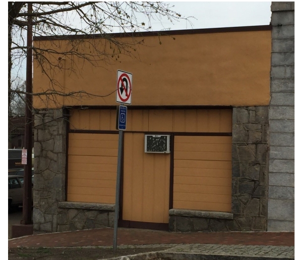
Mothballed building boarded up with yellow plywood.
