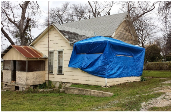
Residential demolition by neglect
