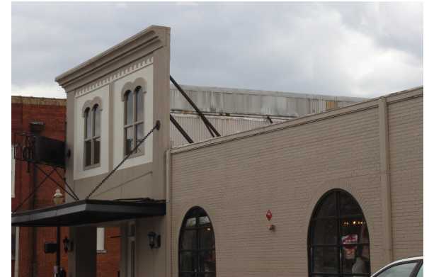
Inappropriate side façade installation that is not original to the building.
