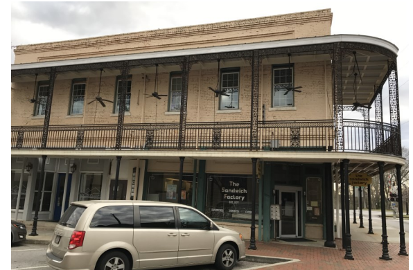
Inappropriate balcony construction not original to building and interrupts sidewalk and storefront activity.
