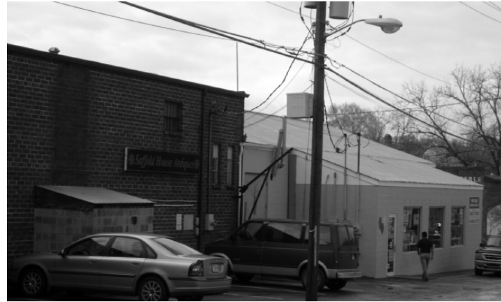
Figure F12 - The gabled roof of this addition to a historic commercial building interferes with the original roofline and detracts greatly from the historic character of the building. The roofing materials are also incompatible with the historic building.
