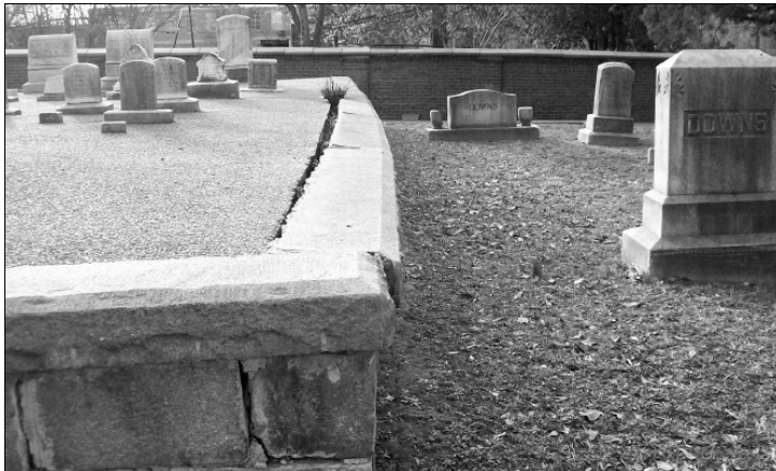
Figure M2 - This raised plot has been paved over in an effort to reduce maintenance, but because a proper drainage system was not established, the walls of the plot are beginning to bow and could soon fall over.
