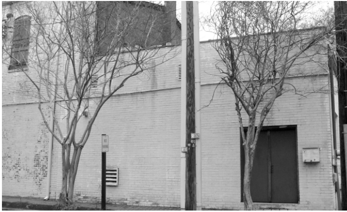
Figure F6 - This is an example of a recommended addition because the materials are like that of the historic building but can be differentiated.
