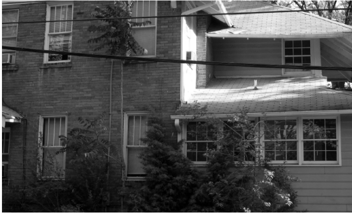
Figure F23—The clapboard addition to this historic brick house is not compatible in many ways, including window type. The 4-over-1 windows present on the historic house are a significant character-defining feature that is diminished by the incompatible 6/6 windows on the addition.
