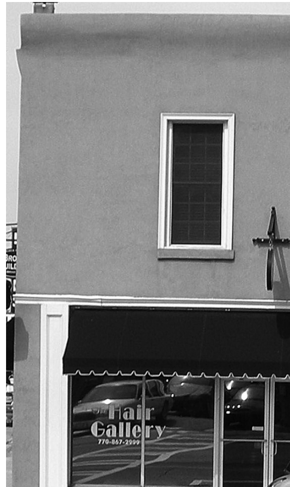
Figure F7 - The addition of an external insulation and finishing system (EIFS) to this historic commercial building is not recommended because it has masked historic materials.
