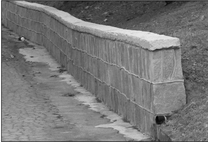
Figure M4 - This retaining wall is made of recommended materials and is located where it will not cause serious drainage issues.
