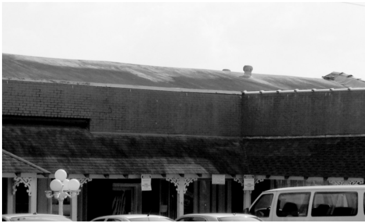
Figure E4 - The roofs of Stone Mountain's historic commercial buildings tend to be built-up or of tar and gravel. These materials should be repaired rather than replaced when maintaining the historic building.
