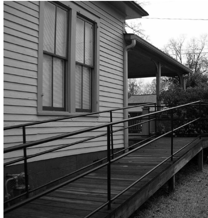
Figure E17 - A ramp has been added to this historic house, but it is located to the side of the main façade and it is screened with shrubs so it does not detract from the historic nature of the house.
