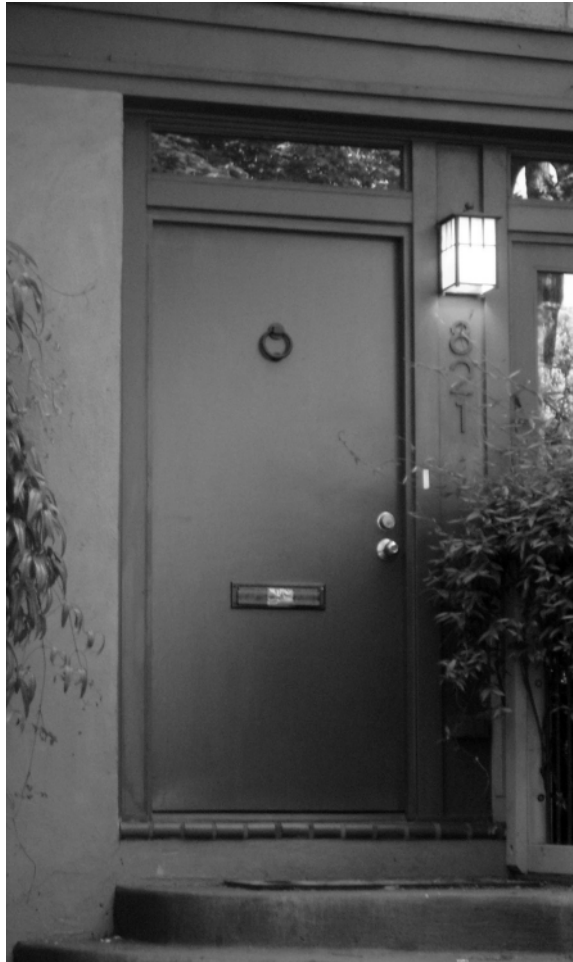
Figure F21 – This flat wood door that does not incorporate glass would be inappropriate on an addition to a house in the Stone Mountain Historic District, since the historic doors of this district most commonly incorporate glass or paneled elements in their design. Doors on additions should be compatible with the historic door types found on the historic building to which the addition is attached.
