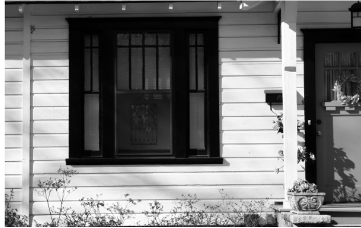
Figure E14 - The wood window of this historic house has been well maintained. The light pattern and materials have been retained although the glass appears to have been replaced with new material.
