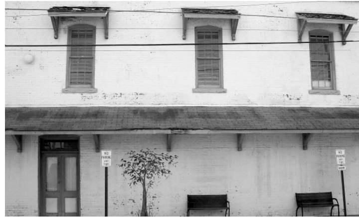
Figure E5 - Awnings such as this should be maintained and repaired, rather than replaced when they exist on historic commercial buildings in Stone Mountain.
