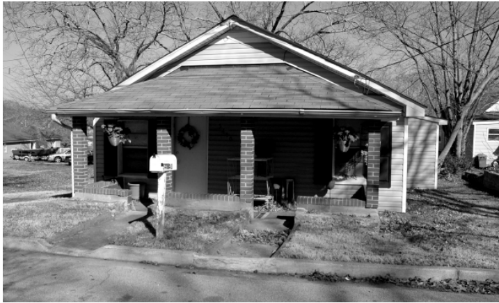
Figure F17 - This addition, made to the right, is recommended because it had been made to the side of the house and the setback allows it to be somewhat hidden from view when looking at the front of the house.
