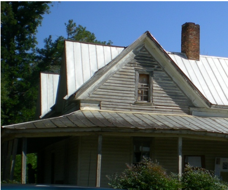
CA Figure 12: Accumulation of debris has resulted in moisture damage to the porch roof. Northwest corner of porch on west facade, facing east.
