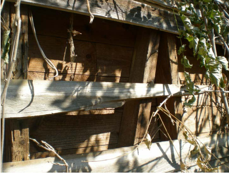
CA Figure 11: Intrusive vegetation and ultraviolet light degradation. Note exposed braced framing and inappropriate repair to siding. South façade facing northeast.
