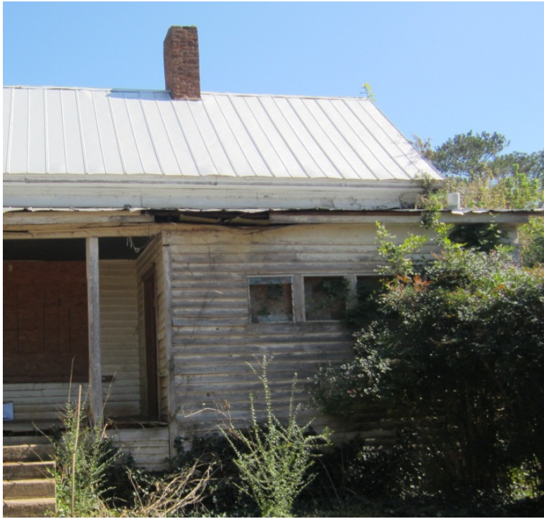
CA Figure 13: Invasive vegetation, west facade, Room 111. Note residual vegetation and black rot to fascia boards.
