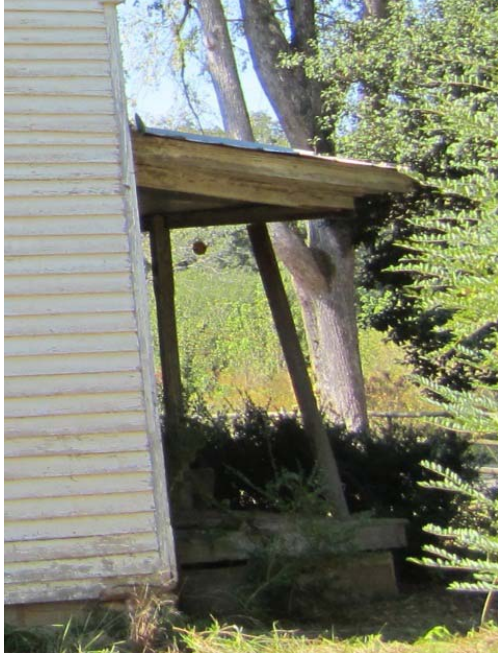
CA Figure 9: Detached column on porch, north facade facing northwest
