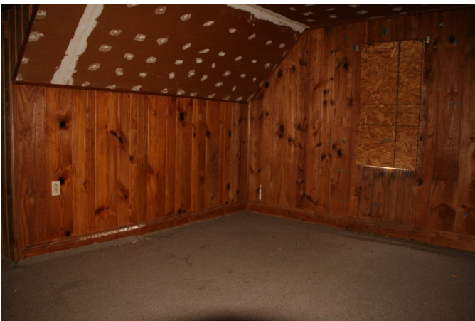
AD Figure 47: Room 203 looking west toward paneled walls and dry walled wall
