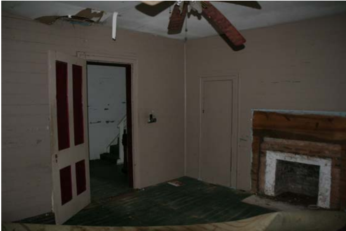
CA Figure 23: Room 104-Damaged ceiling due to water damage
