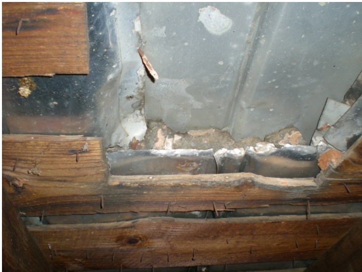
CA Figure 4: Inappropriate roof repair as viewed from the attic facing east.
