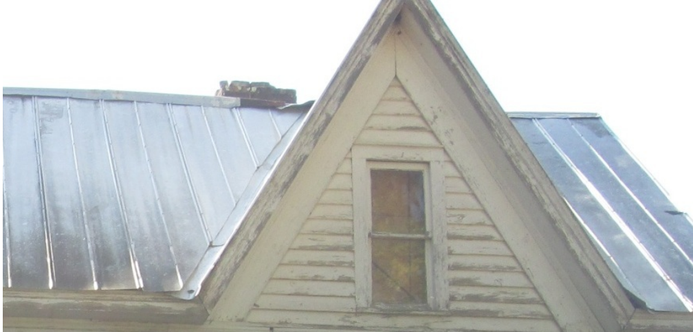
CA Figure 1: Damage to ridgecap, west corner of north facade, facing south.
