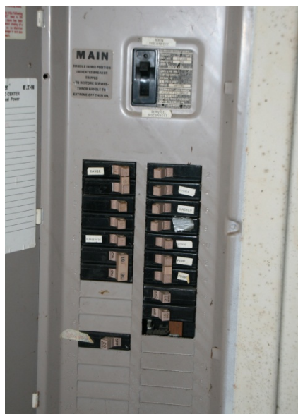
AD Figure 53: Circuit Breaker in room 107
