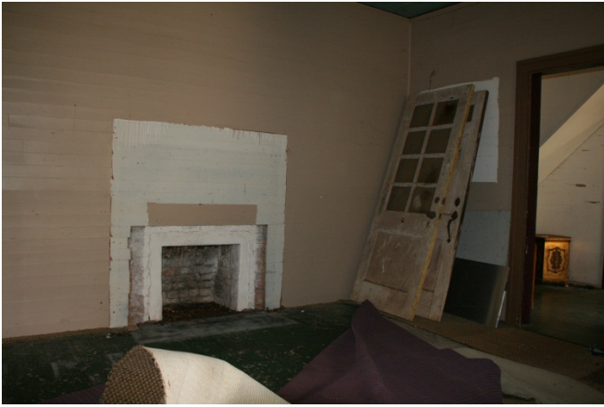
AD Figure 15: Missing mantel from fireplace in Room 101
