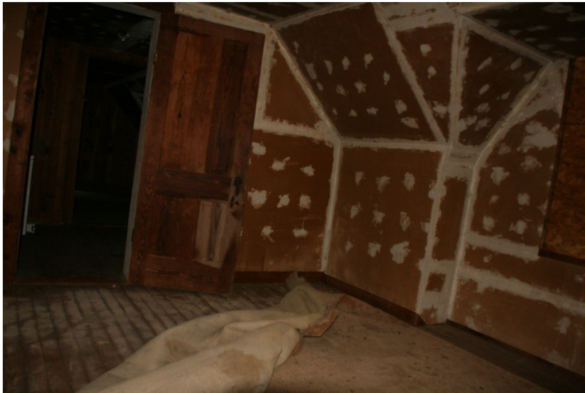
CA Figure 30: Room 201-Door D19 with matte finish on stain, worn carpet, typical drywall condition, and missing pieces of baseboard.
