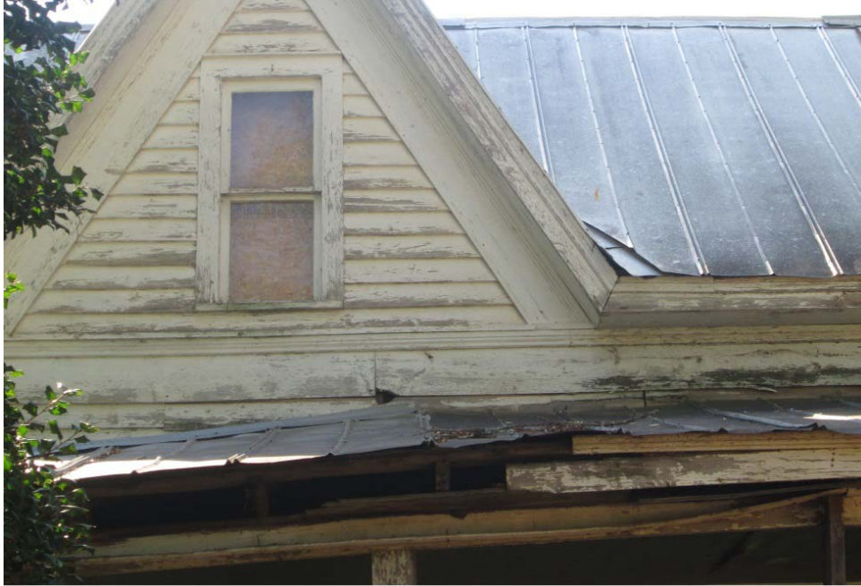
CA Figure 7: Brown rot on the fascia board of porch; northeast corner of porch, north facade.
