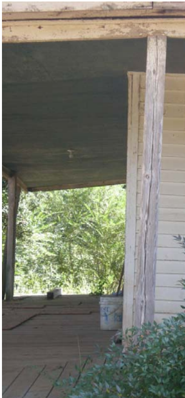
CA Figure 8: Floor boards have been replaced with plywood. Note leaning columns and differing sizes of floor boards. Northwest corner of building facing east.
