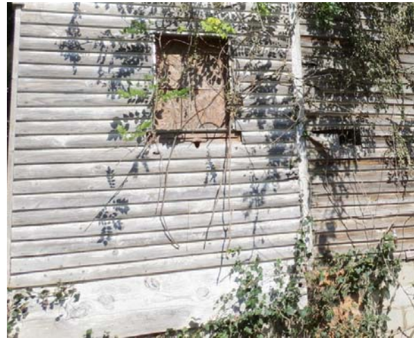
AD Figure 10: Variation in the paint color and the change of the clapboard siding on south façade
