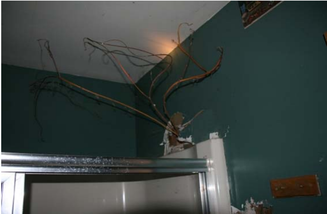
CA Figure 25: Room 106-Vegetation growing through a hole in the east wall
