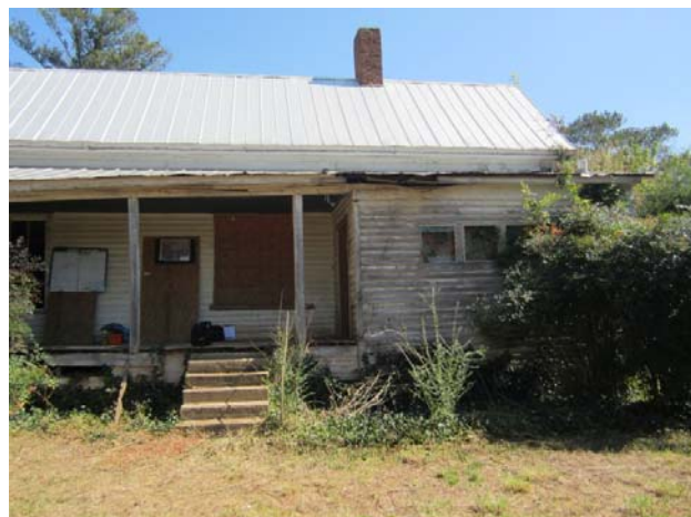
AD Figure 12: Set of concrete stairs on the west facade of Sherrill House
