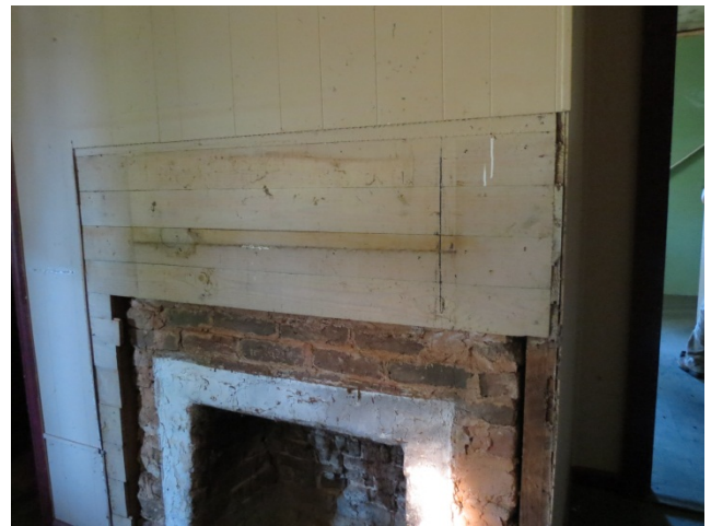
AD Figure 28: Fireplace in Room 105 that is missing mantle
