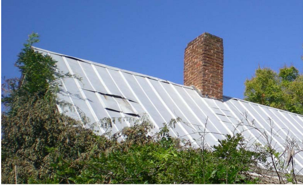
CA Figure 3: Inappropriate repair to roof enables water to enter building. East façade along exterior of room 109, facing northwest.
