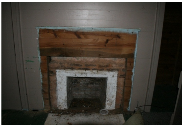
BC Figure 3: Fireplace in Room 104 that is missing a mantel
