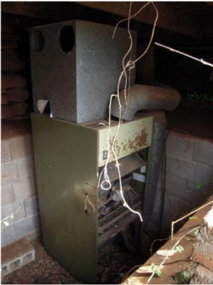
AD Figure 57: Furnace underneath the south crawlspace of the house
