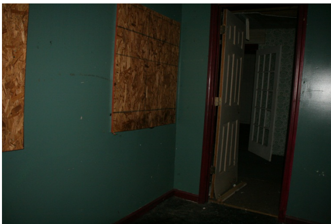
AD Figure 29: Room 106 looking west toward D12 and windows W9 and W10
