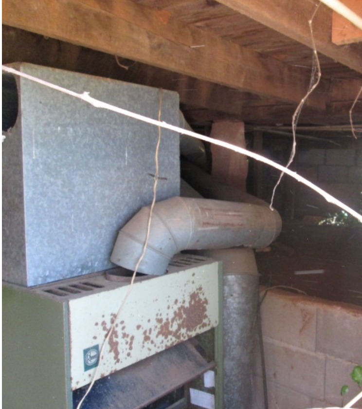
CA Figure 17: Heating unit and disconnected ventilation ducts. In crawlspace facing northeast.
