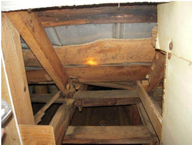
AD Figure 3: Remnants of wood shingles and underlying sheathing with visible nails
