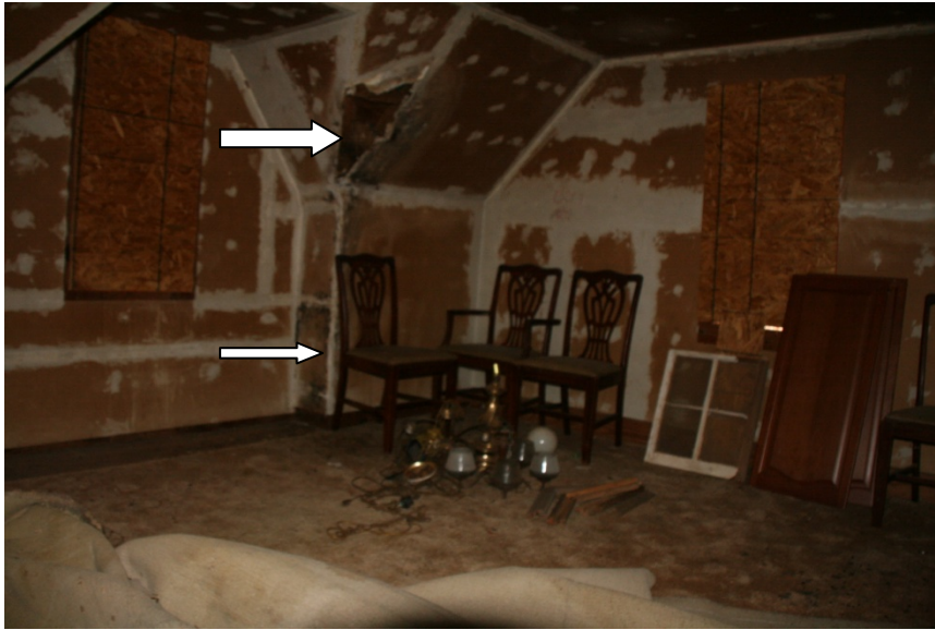
CA Figure 29: Room 201-Top arrow denotes hole in drywall with accumulated debris. Bottom arrow denotes black mold growth from water leak.
