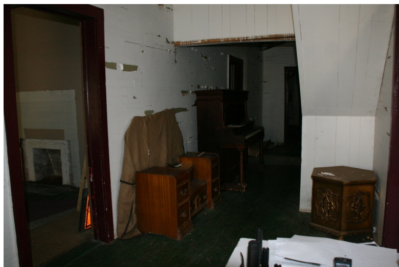
Room 102 and peeling Latex paint on walls
