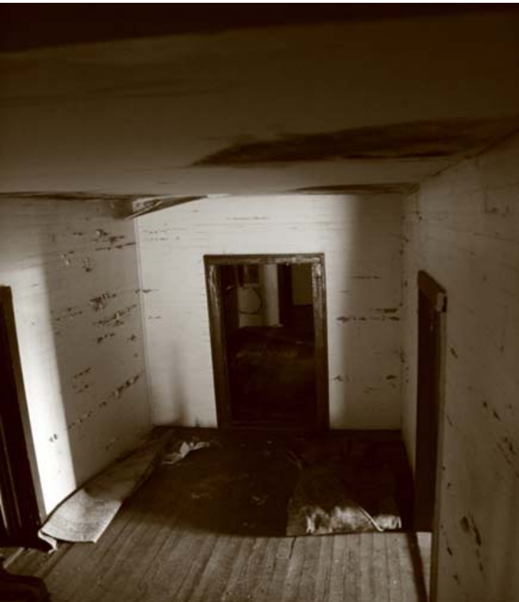
CA Figure 20: Room 102-Water damage/mold on ceiling, peeling paint on walls
