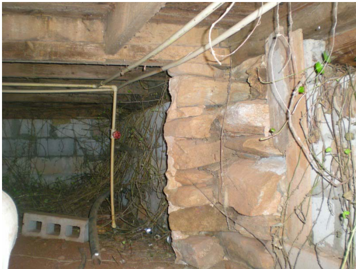
CA Figure 6: Stacked stone, PVC pipes, and CMU infill under Rooms 109 and 110 facing east. Note black rot along sill where vegetation is encroaching.
