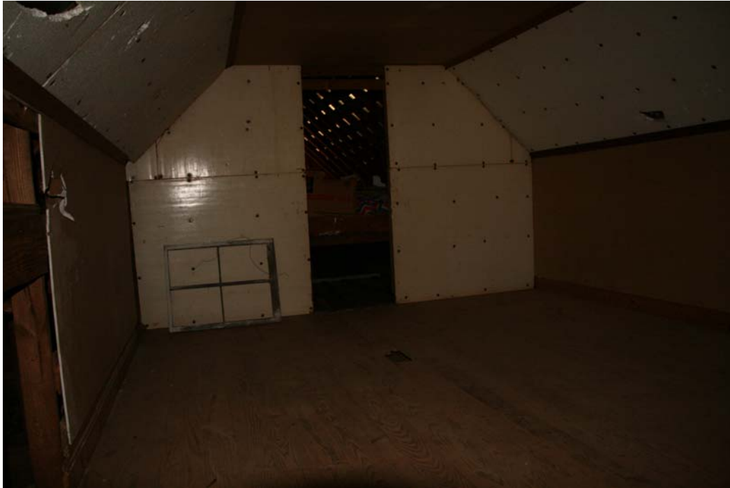
CA Figure 33: Room 205-Significant damage from roof leaks has damaged the insulation panel in this room and caused water and mold damage in Rooms 102 and 105 below.
