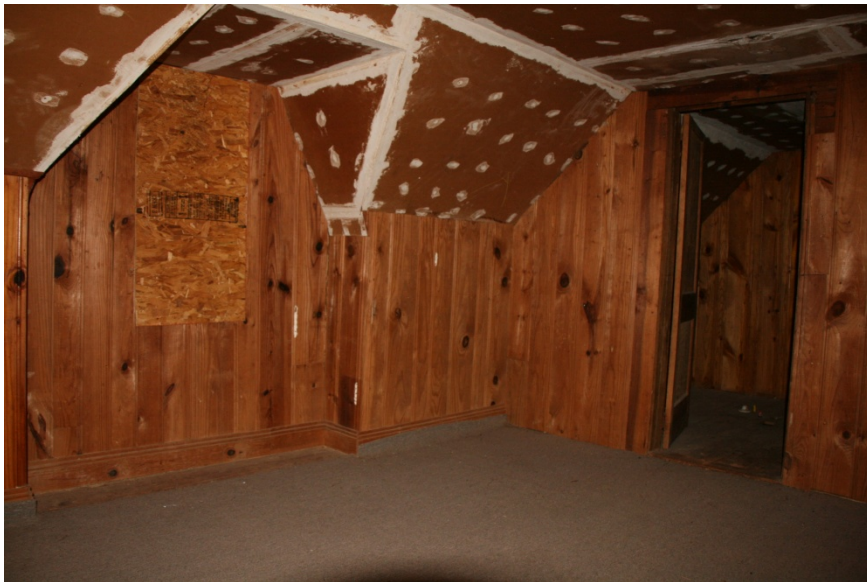
CA Figure 32: Room 203's level of finish and condition is better than those observed in Rooms 201 and 202.
