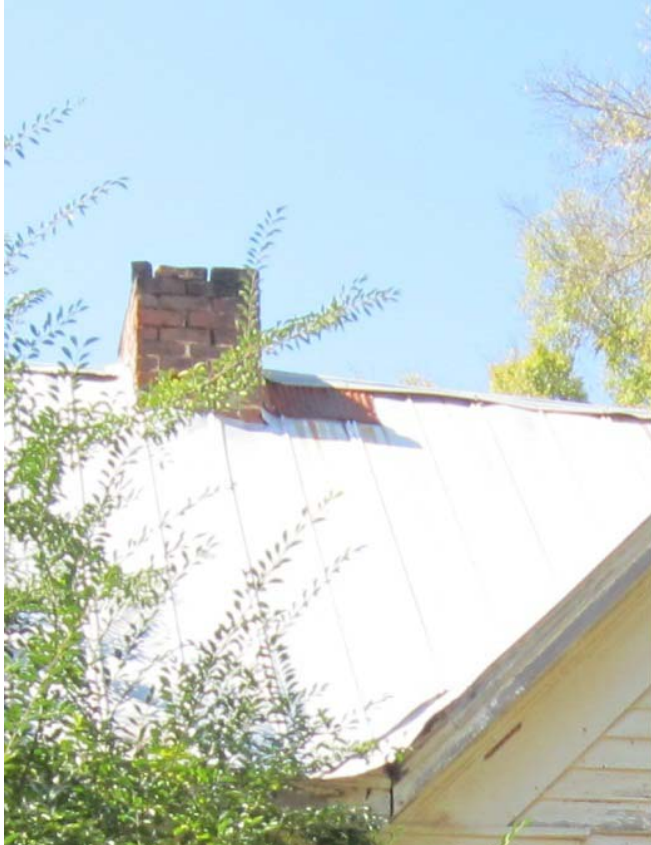
CA Figure 5: Damage to ridge cap and flashing east façade facing northwest. Note galvanic corrosion to repair and lack of flashing around to chimney.
