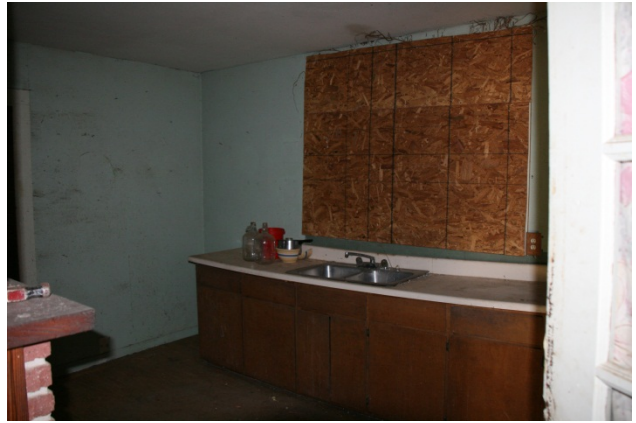
AD Figure 56: Sink area on the south wall of Room 110
