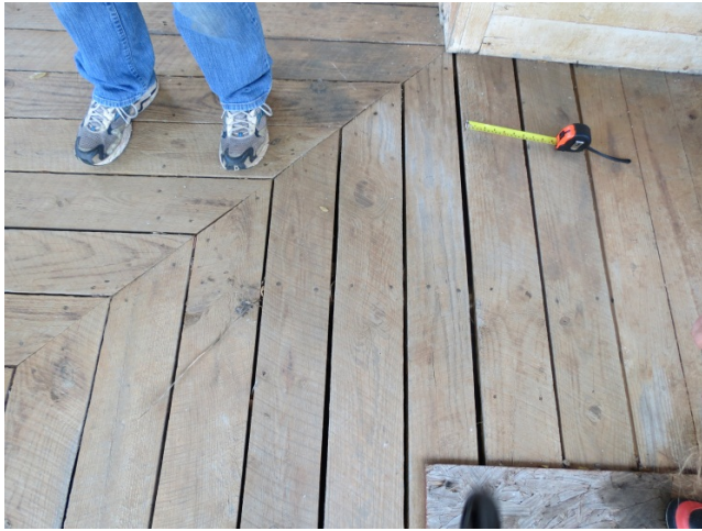
AD Figure 1: The floor of the porch is comprised of wood plank floorboards
