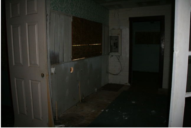
AD Figure 31: Room 107 looking south at the circuit breaker toward Room 109
