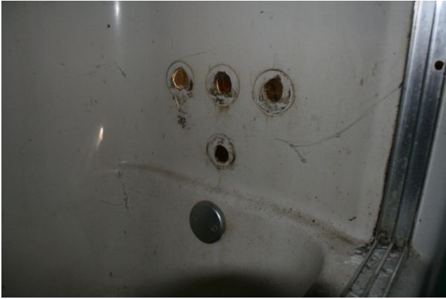
AD Figure 55: Missing fixtures in the shower in Room 106
