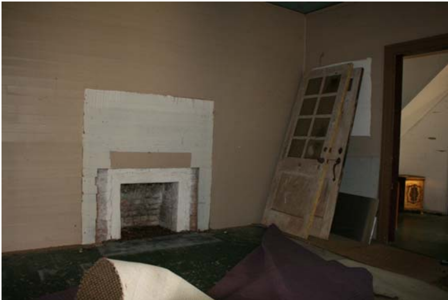
CA Figure 18: Room 101- Missing mantel, tongue and groove flooring under carpet
