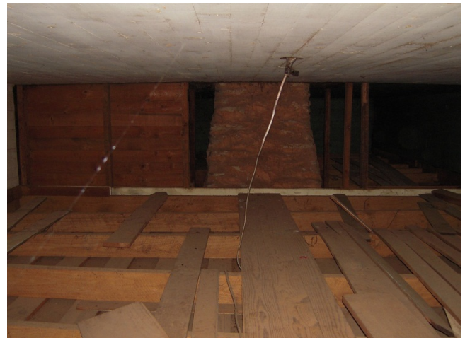
AD Figure 52: Dropped ceiling and electrical wires over room 108
