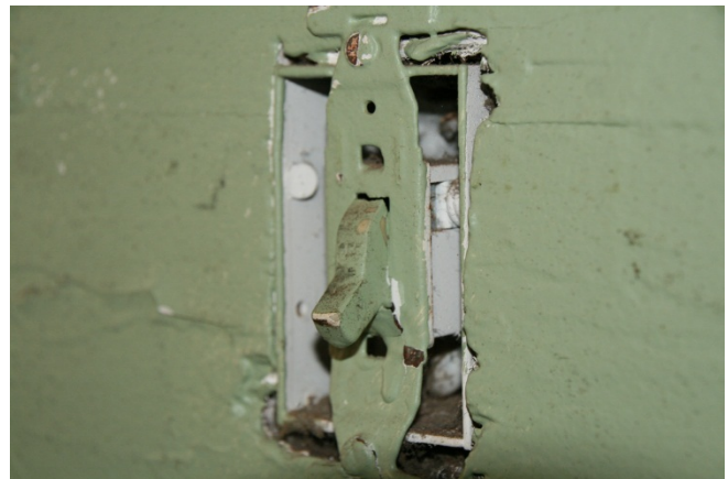
AD Figure 54: Electrical Switch in Room 109
