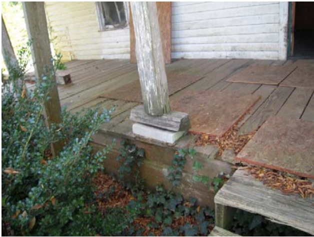
AD Figure 7: Unstable porch column on the North Facade by front door
