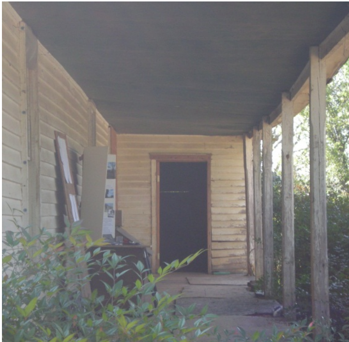
CA Figure 14: Facing south from NW corner of north facade along porch. Note loose siding and missing floorboards repaired with plywood.
