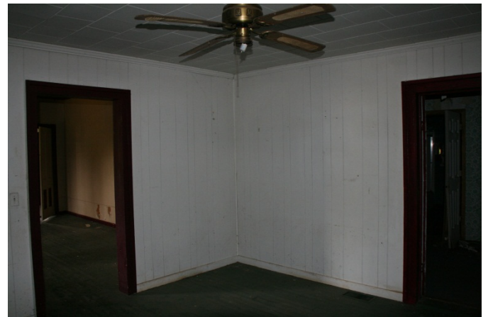
AD Figure 36: Room 108 looking southeast, door to Room 107 is to the right
