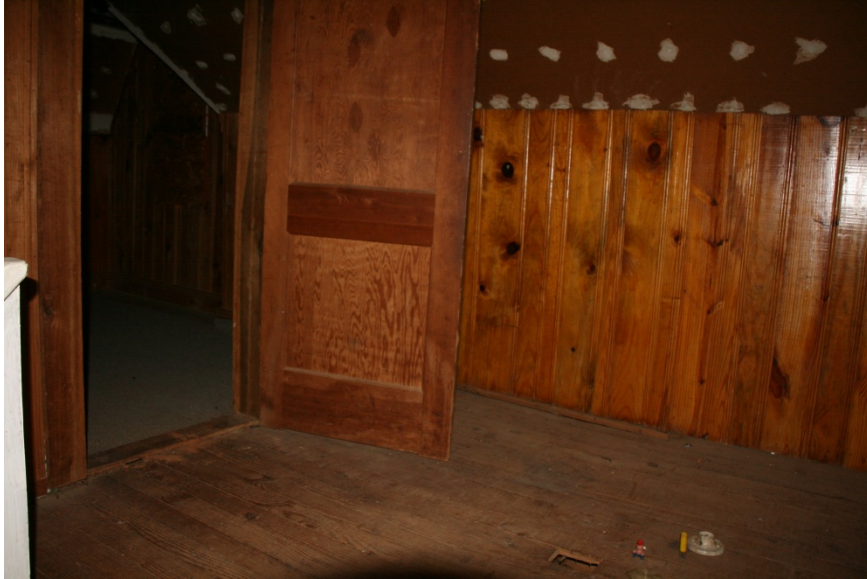
CA Figure 31: Room 202-Door D22 without high gloss stain prominent against high-gloss finish on north wall behind it. Bottom center of picture shows the hole in the floor to access ceiling light in Room 102.
