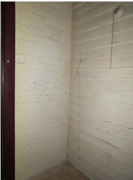
AD Figure 39: Exterior siding that now serves as a wall to Room 107
