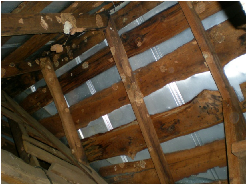
CA Figure 2: Black rot on roof sheathing due to ridge cap damage. Mud daubers nests are present on the sheathing and rafters. North end of attic facing northeast.
