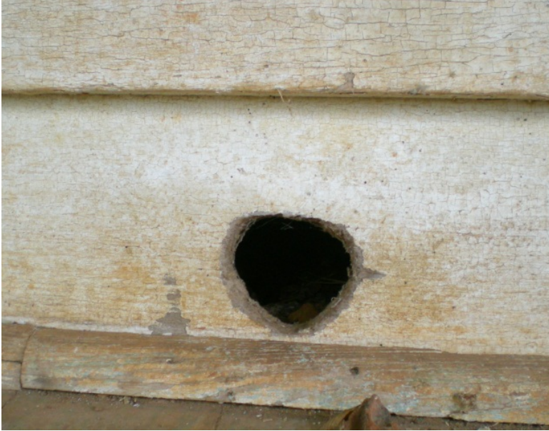
CA Figure 15: Hole in siding due to presence of rodents or other pests; west facade along porch, facing east.
