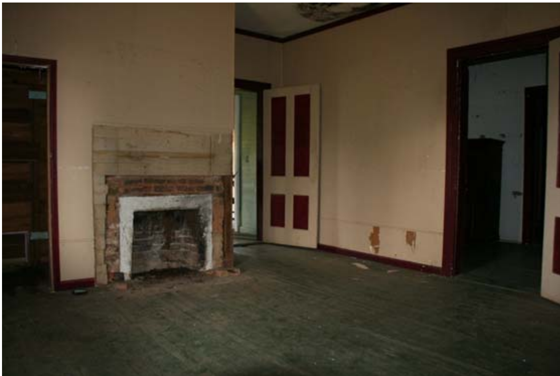
CA Figure 24: Room 105-Missing mantel; tongue and groove flooring
