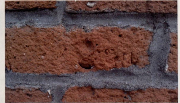
This image of disintegrated brick shows the damage that can be caused by abrasive cleaning techniques like sandblasting.
