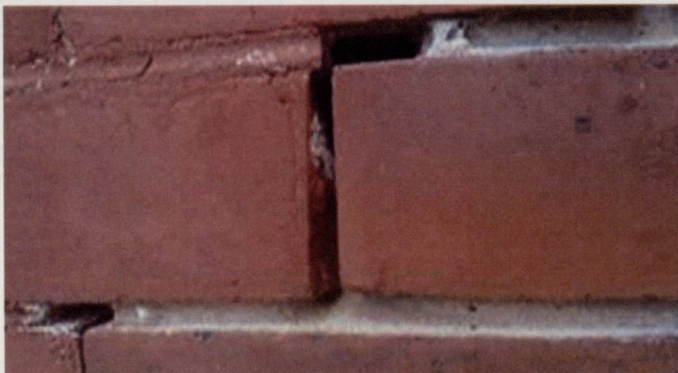
An example of damaged mortar joints.
