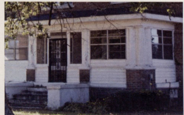
This porch enclosure is inappropriate because it was done using opaque siding materials that heavily alter the porch's historic look and use.
