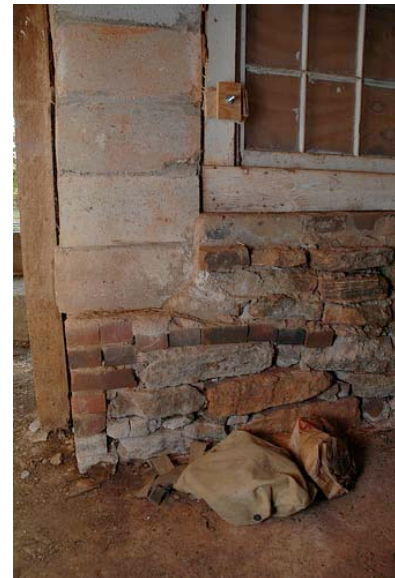
Fig. III-42. Southwest wall of Room 001, showing brick and CMU infill in the granite wall.
