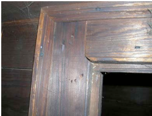
Fig. III-131 Door frame to Room 201. Door is missing therefore not numbered.
