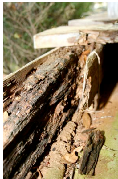
Fig. IV-43. Outside sill of the west porch damaged by water and possibly termites.
