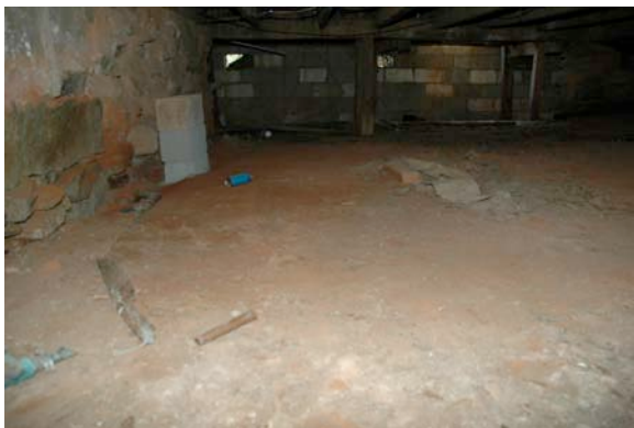
Fig. III-38. Overview of the foundation looking to the west. To the south is the granite wall of the basement (Room 001). To the west is the CMU foundation of the west porch.
