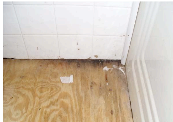
Fig. IV-62. Water damage on plywood subfloor, Room 103.
