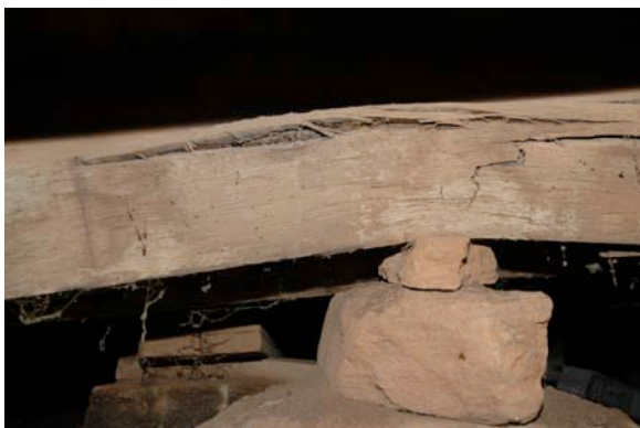
Fig. IV-25. Looking east, showing damage to the summer beam.
