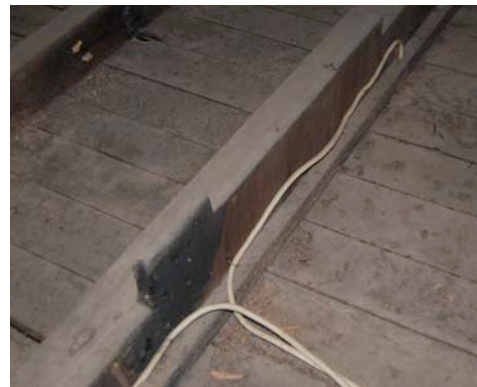
Fig. III-77. East wall of stairwell extends into the main house attic at the eighth ceiling joist from the access panel (going west to east). The wall is constructed of tongue-and-groove vertical panels. There appears to be some fire damage.
