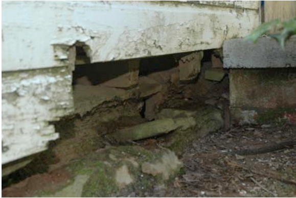
Fig. IV-23. Termite damage to sill on north facade.
