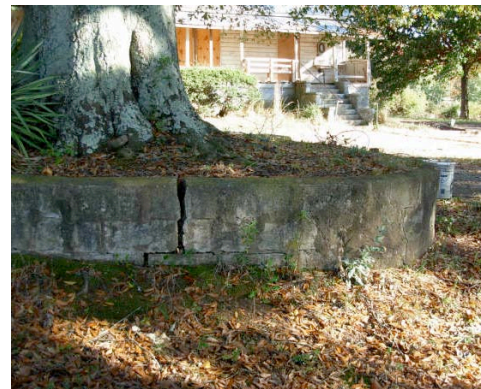
Fig. III-7. Looking east. CMU area of retaining wall; tree roots causing cracking.
