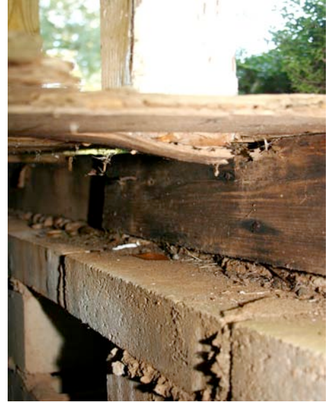
Fig. IV-45. Close up of one of the supports next to the hole in the west porch. Note the deterioration under the floor where the post is not supported.
