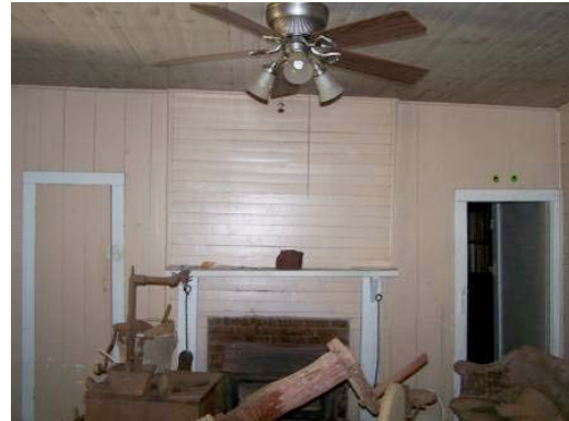
Fig. III-112. Room 106. Brushed chrome fan with light fixtures.
