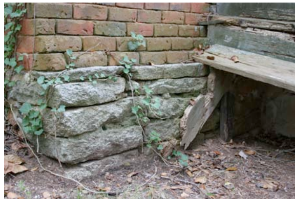
Fig. IV-36. Foundation of west chimney. Notice the missing mortar on the foundation and the bricks above. Also seen are the damaged north steps.
