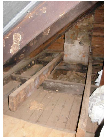
Fig. IV-71. Chimney flue in attic (Room 207) rests on a piece of sheet metal used to patch the ceiling in the kitchen (Room 107) below.
