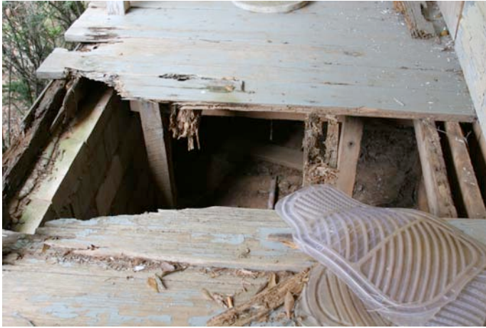
Fig. IV-40. Hole in the west porch due to water and termites.
