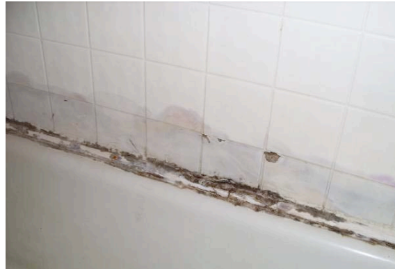
Fig. IV-63. Mildew at tub-tile panel intersection, Room 103.
