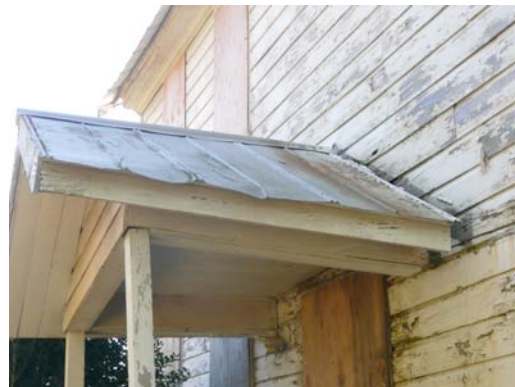
Figure IV-30 Portico (North facade). Notice detachment from house.
