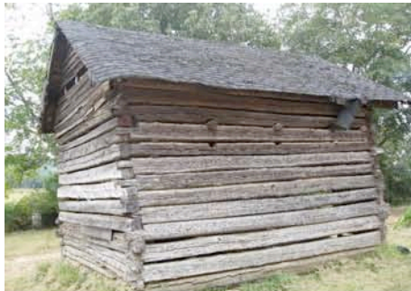
Fig. III-9. East gable end and north facade of the smokehouse. Notice the ends of the two logs projecting from the north facade as well as the loose asphalt shingles and the
