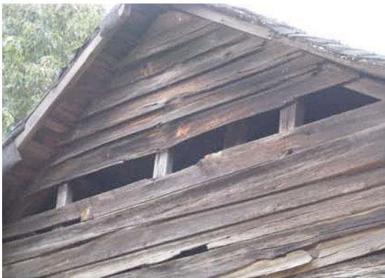
Fig. IV-6. Ultraviolet damage to the east gable end of the smokehouse. Notice that some of the boards have started to buckle and that others are missing.
