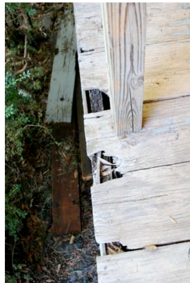
Fig. IV-39. Deterioration at the edges of the porch due to water.
