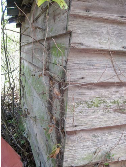
Fig. III-19. Northwest corner of the single pen. Notice the lack of corner boards.
