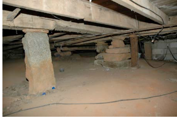
Fig. III-39. Overview of the foundation, looking northeast. To the west is a large granite block pier. To the east is a stacked granite pier that has been reinforced with a wooden block. At the far, east side is the CMU foundation of the eastern porch.
