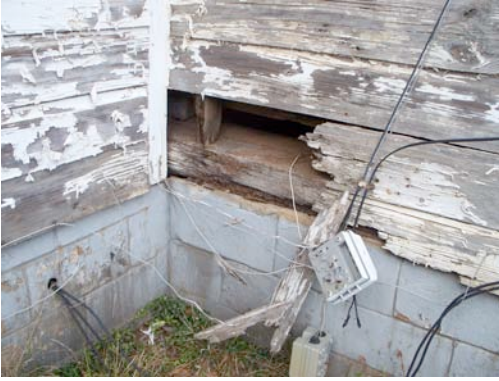
Fig. IV-55. Hole in siding just above foundation.
