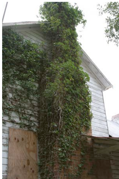
Fig. IV-32. West chimney covered in vines.
