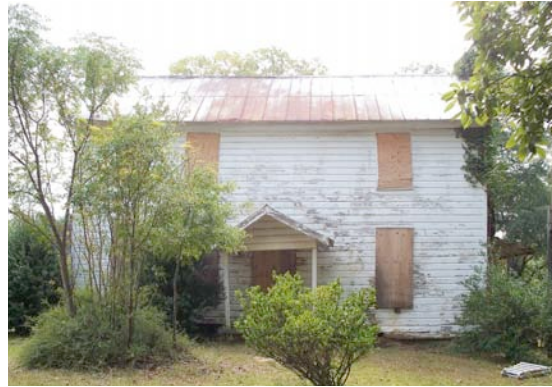
Fig. III-75. North façade of the main house with side-gabled roof with standing-seam, galvanized steel roofing. Note the metal corrosion.
