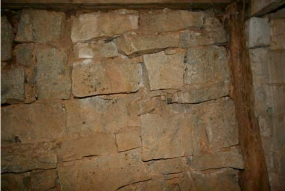
Fig. III-60. Wide view of the granite steps from under the porch. Note the support to the right that separates the CMUs and the granite. It is believed that these are the original steps up to the log cabin (ca. 1850).
