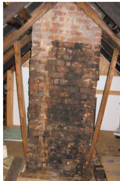
Fig. III-83. Attic (Room 207). Central interior chimney. Notice the creosote buildup on the exterior of the chimney.
