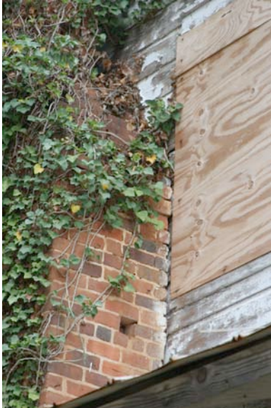
Fig. III-51. One of the missing bricks on the west chimney, south side of the chimney next to window W21.
