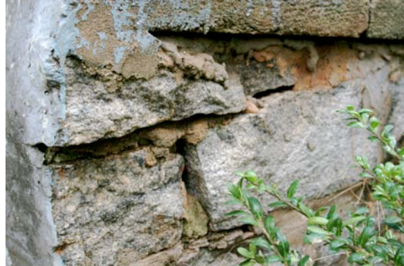
Fig. III-61. Close up of the side of the main stairs. Note the repointing of the stones.
