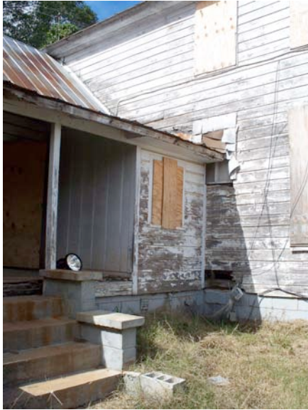
Fig. III-67. Junction of main house and ell, showing hole in wall cladding.
