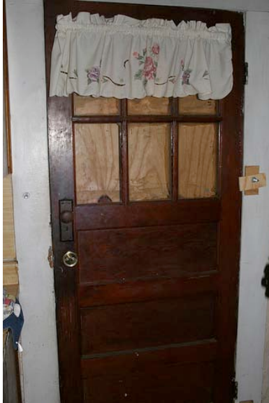
Fig. III-118. Room 107. Door (D14) on west side.
