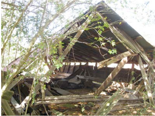
Fig. IV-18. What remains of the east facade of the small barn.
