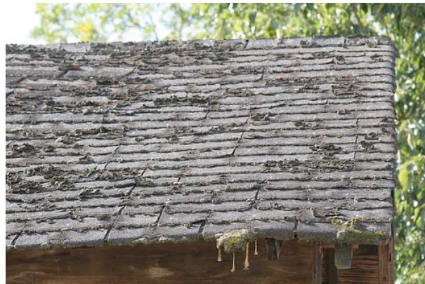
Fig. IV-7. Deteriorating asphalt shingles on the north plane of the smokehouse roof
