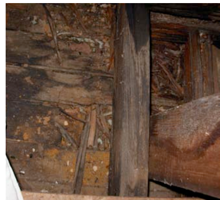
Fig. IV-58. Attic (Room 207). Rot and water damage around the south interior chimney affects the ceiling joists and the wood that forms the ceiling.
