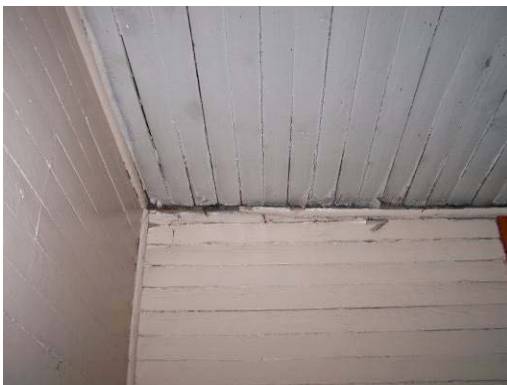
Fig. IV-69. Room 106. Northwest corner has moisture damage and missing shoe molding.
