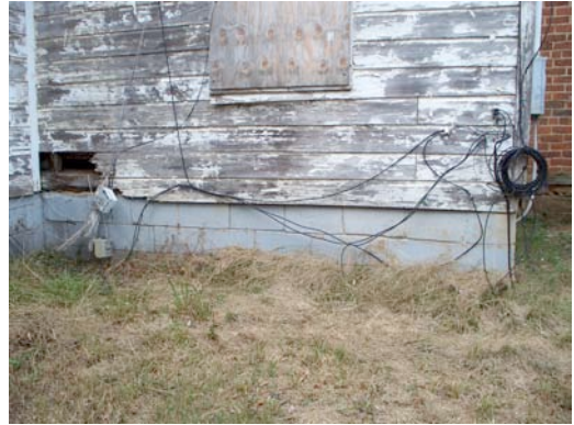
Fig. IV-48. CMU foundation on the east façade.
