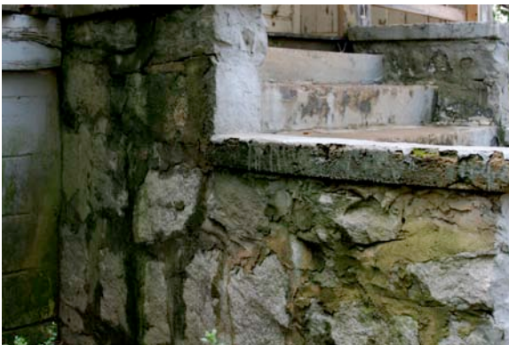
Fig. IV-38. Close-up of the north side of the main stairs. Notice the repointing with portland cement.
