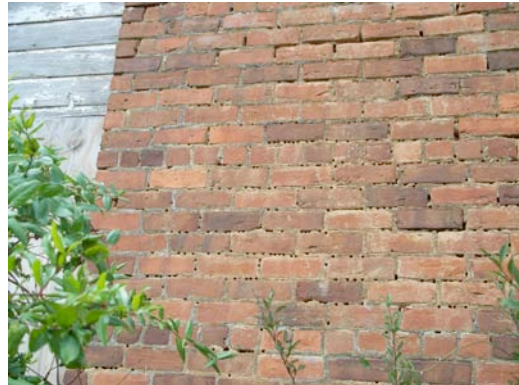
Fig. IV-52. Holes in east façade chimney created by birds.
