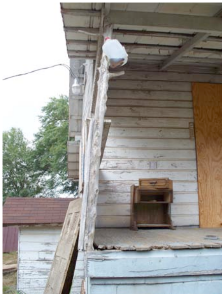
Fig. III-74. Tree branch as porch support on east façade.
