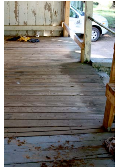
Fig. III-57. Floor of the west porch. This is the south end of the porch where the floor appears to have been recently replaced.
