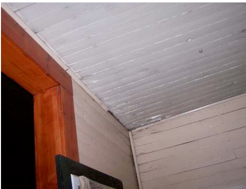
Fig. IV-68. Room 106. Northeast corner has missing shoe mold.
