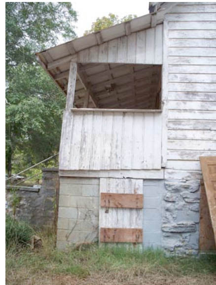
Fig. III-66. Detail of western section of south foundation, showing CMU and granite foundation.
