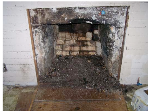
Fig. III-116. Room 107 fire place revealed, whitewashed granite hearth surround. One of the fireplaces of the original saddlebag house.
