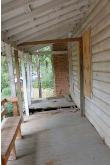
Fig. III-54. West porch looking north. Notice the large hole in the porch.
