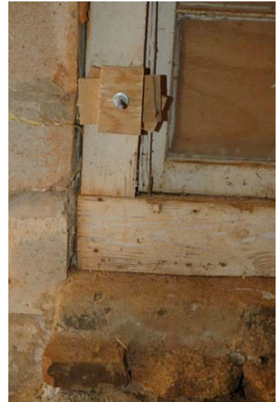
Fig. IV-27. Close-up of window W2 showing damage to frame due to bolted-on plywood.
