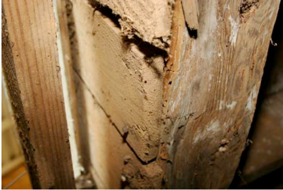
Fig. III-64. Evidence of siding material under the existing siding. Viewed from the hole in the west porch.
