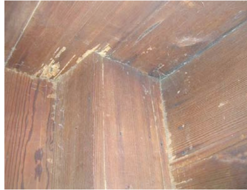
Fig. IV-75. Termite damage to northwest corner Room 203.
