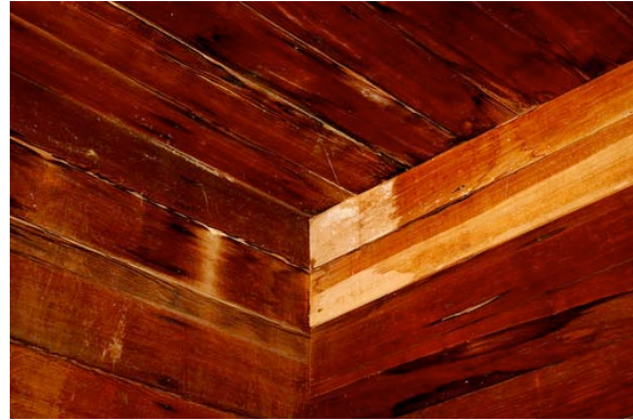
Fig.IV-61. Water damage at ceiling and upper walls, Room 102.
