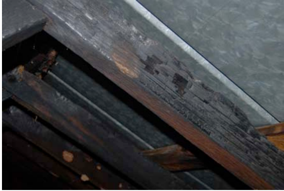
Fig. III-78. Fire damage to rafters in main house attic.
