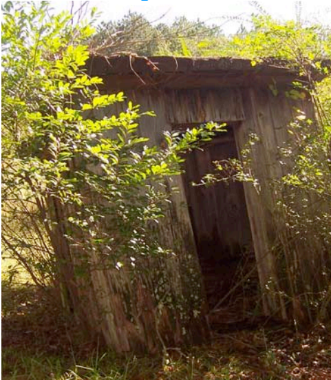
Fig. IV-2. Vegetation encroaching on privy.
