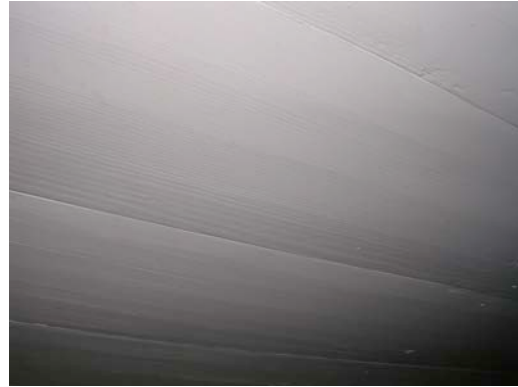
Fig. III-135. Ceiling boards in Room 205 showing hand-planing marks running longitudinally along the length of the board.
