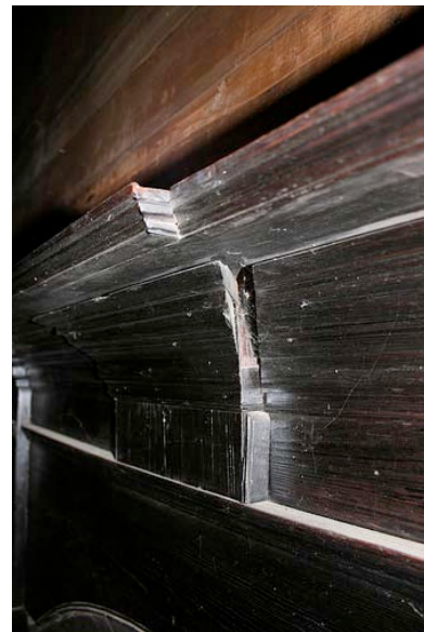
Fig. IV-66. Missing wood trim at fireplace mantel, Room 105.
