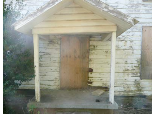
Figure IV-29 Portico (North facade). Notice leaning columns.
