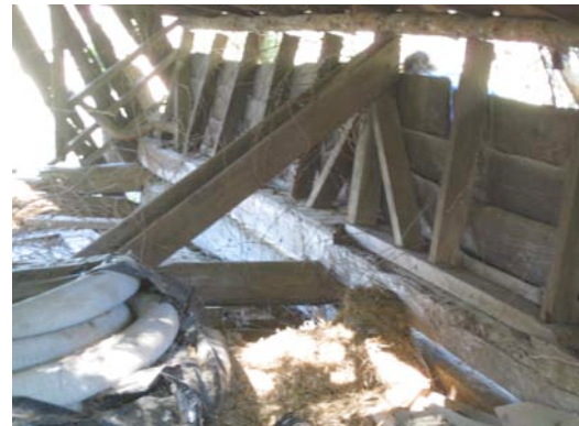
Fig III-29. Interior north wall of the small barn. Notice the braced frame members as well as the hand-hewn tree log acting as the plate.
