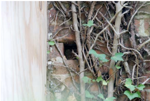
Fig. III-52. Another of the missing bricks on the west chimney, north side of the chimney, note the lack of mortar in the space.
