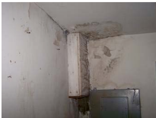
Fig.IV-64. Room 104 . Moisture around fuse box.
