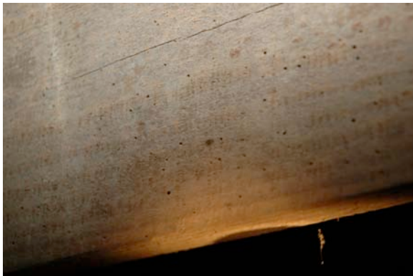
Fig. IV-24. Powderpost beetle damage to south sill.
