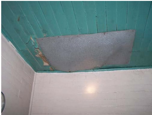
Fig. III-122. Room 107, ceiling patch, where chimney or flue is subsiding.
