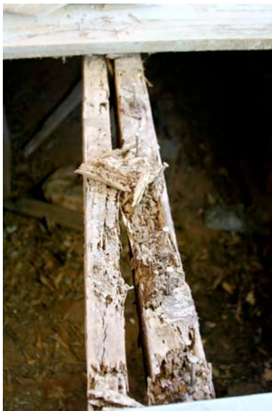
Fig. IV-42. Damaged porch support due to termites.
