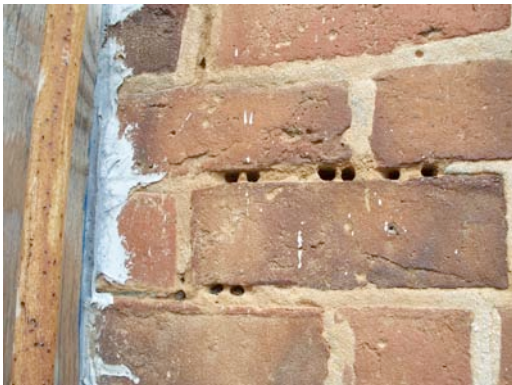
Fig. IV-53. Detail of bird holes in east façade chimney.
