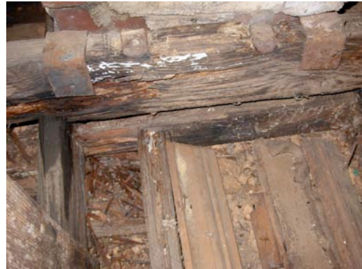
Fig. IV-57. Attic (Room 207). Lack of chimney crickets around the south interior chimney has caused the wood around the chimney to rot. The two metal bars and the joist are used to defer the weight of the chimney from the ceiling to the joist. However, the rot has caused this system to fail and the weight of the chimney now rests on the ceiling.
