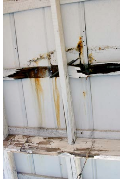
Fig. IV-41. Roofing above the hole in the west porch. Note the rust and damaged wood supports. There are also several small holes in the material.
