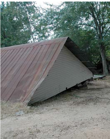
Fig. III-27. Close up of the collapsed garage.
