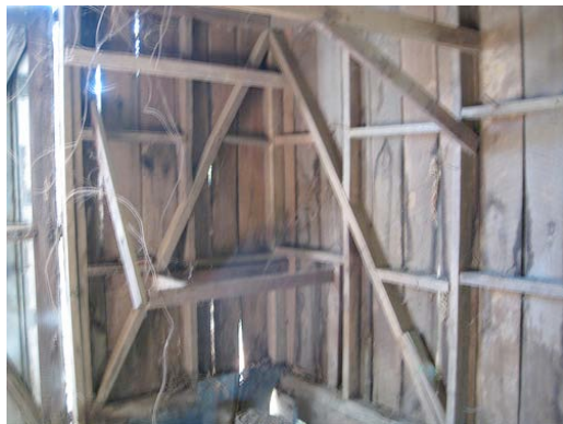
Fig. III-14. Southeast corner of the workshop. Notice the diagonal boards forming the “brace” in braced frame construction.
