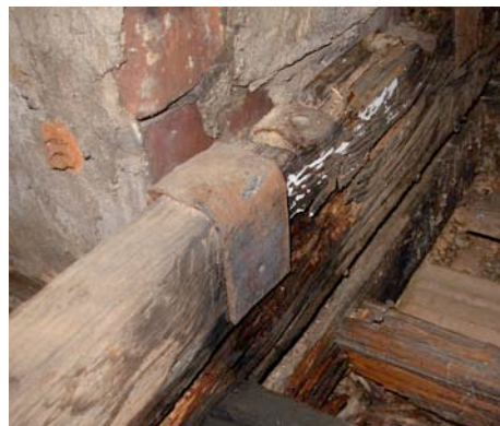
Fig. III-85. Attic (Room 207). Metal over joist to help defer chimney's weight from the ceiling to the support joist.
