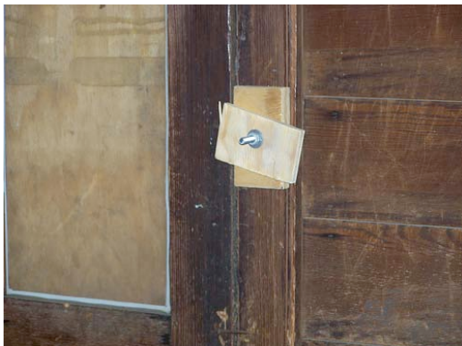
Fig. IV-60. Example of damage to wood frames, Room 105, a result of measures taken to secure the house openings.
