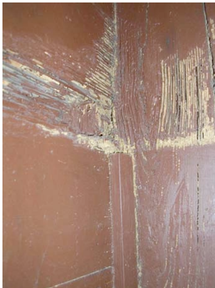
Fig. IV-74. Termite damage to paneling, Room 205.
