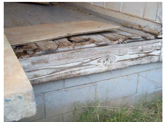
Fig. IV-50. Deterioration of wood floorboards on East Porch.
