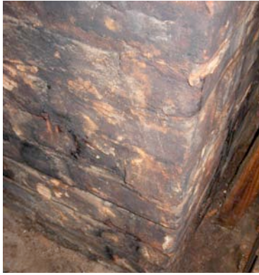
Fig. IV-59. Attic (Room 207). Buildup of creosote on the exterior bricks of central interior chimney. This buildup suggests that there is a crack or opening in the flue.
