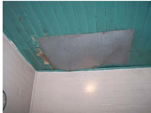
Fig. IV-70. Room 107, ceiling patch, where chimney or flue is subsiding.
