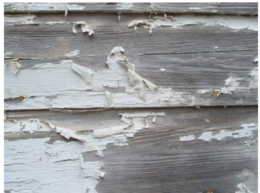
Fig. IV-49. Paint deterioration on the east façade
