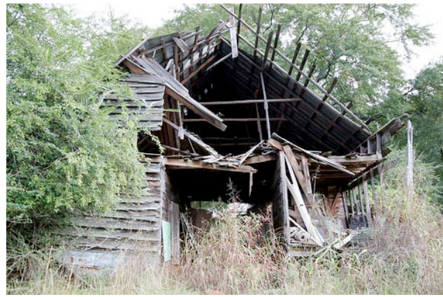
Fig. IV-16. What remains of the west façade of the barn.
