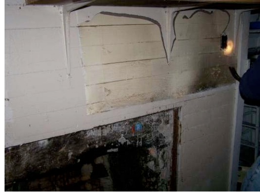
Fig. III-115. Room 107, patch pulled away to reveal original board siding.
