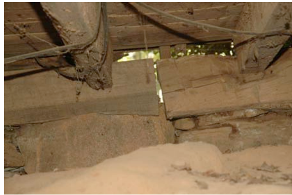
Fig. III-44. View of the central north foundation showing abutment of sill pieces. The sill on the left is circular sawn; the sill on the right is hand-hewn, indicating that the left sill is a replacement.
