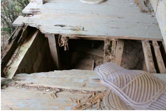
Fig. III-58. Hole in the west porch. Notice the damage to the supporting structures.
