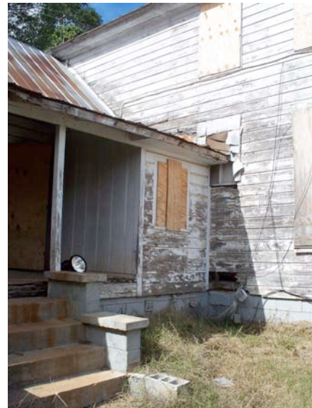
Fig. IV-47. The junction of the east façade with the south façade of the I-house, showing damage to the siding.
