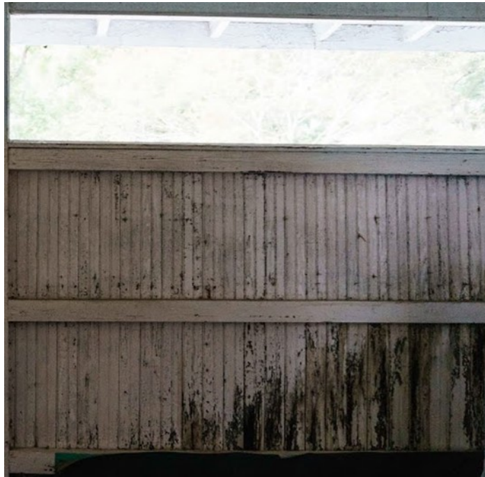
Figure 94. Rot on lower section of the west wall of Room 207.
