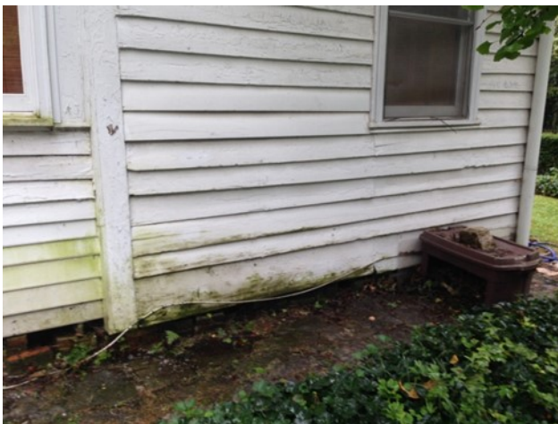
Figures 116-117: North Façade gutter system failure on the kitchen addition
