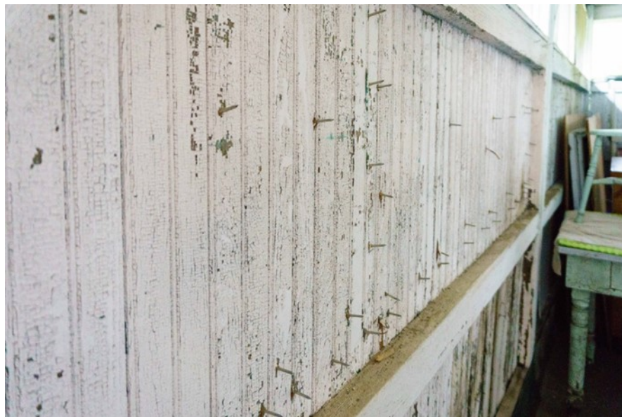
Figure 95. Nails protruding through the bead board on the west wall in room 207. Some alligatoring is also evident.
