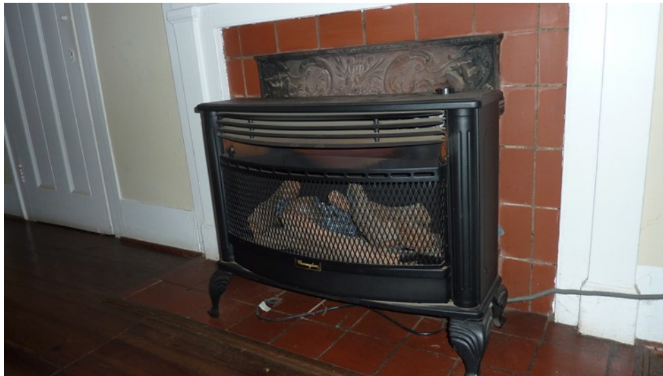
Figure 99. Current gas-powered heaters, like this one in Room 103, block historic hearths from view and can be dangerous if touched.
