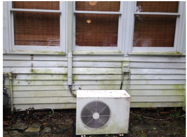
Figure 111: West Façade with microclimate visible underneath exterior windows.
