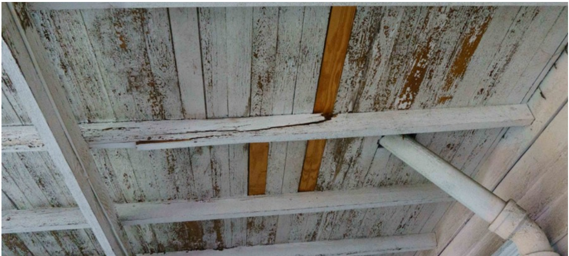
Figure 97 Cracked rafter in Room 206.
