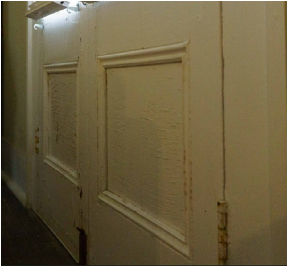
Figure 84. Crazing on the lower panels of the double doors on the east wall.
