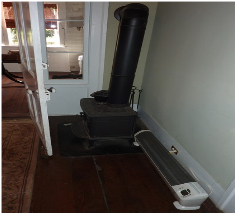
Figure 58. A wood-burning stove and electric radiator in Room 105 are two examples of heating systems present in the house.
