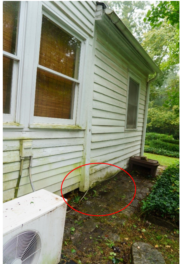
Figure 76. Gutter sagging and leaking. Note accumulation of mildew on the siding due to the water leaking from the gutter.
