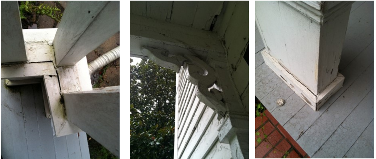
Figures 113-115: East Façade porch columns and brackets are broken
