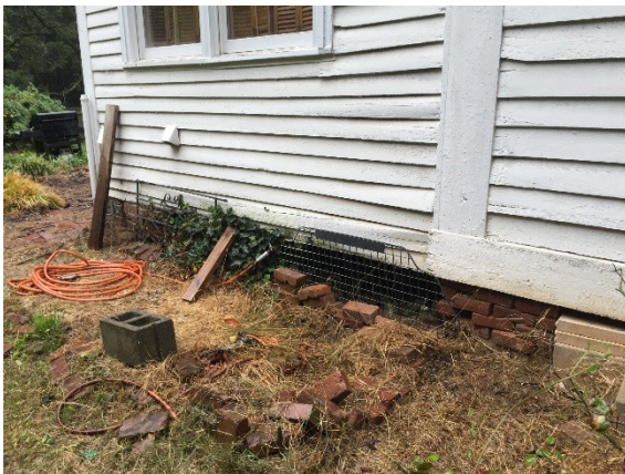
Figure 69. Brick foundation pier with deteriorated mortar
