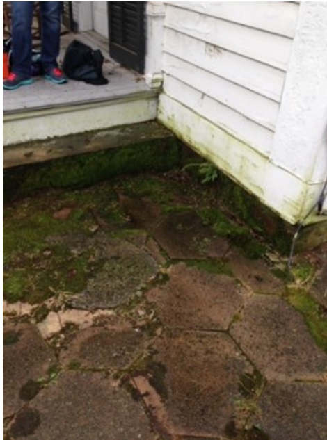
Figure 108 East façade on northeast corner microclimate visible due to excessive water.
