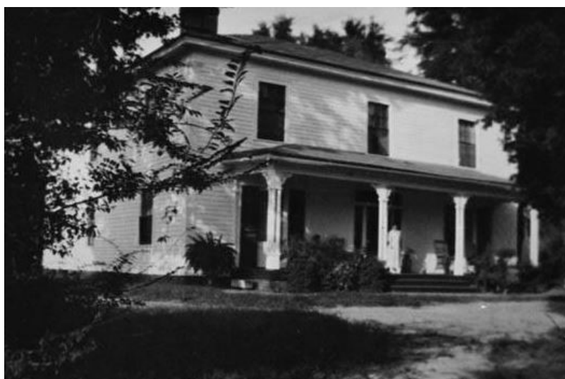
(Left) Figure 1. Evidence of former hipped roof in attic space (Right) Hipped roof on main house and front porch, ca. 1910-15 Photo courtesy Vanishing Georgia Archives
