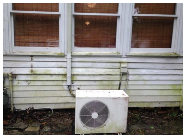
Figure 106. Moisture causing algae staining on the east side of the central addition.
