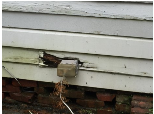
Figure 104. Wood rot on the west façade of the house, south of the back door. (This has been repaired since the initial conditions assessment site visit was conducted.)
