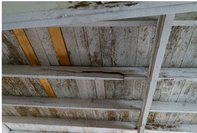
Figure 138: Room 206 roof rafter cracked.
