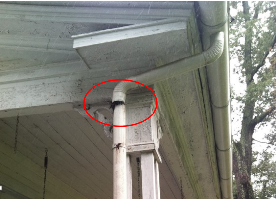
Figure 75. Downspout not connected and leaking.
