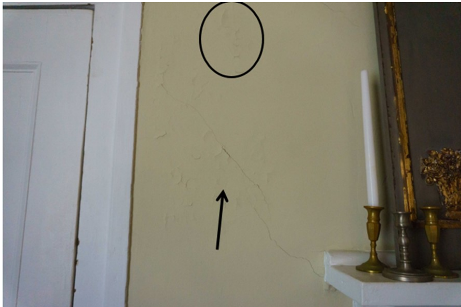
Figure 82: East wall in room 103. Note the crazing in the circle and the arrow pointing to the cracks in the plaster.
