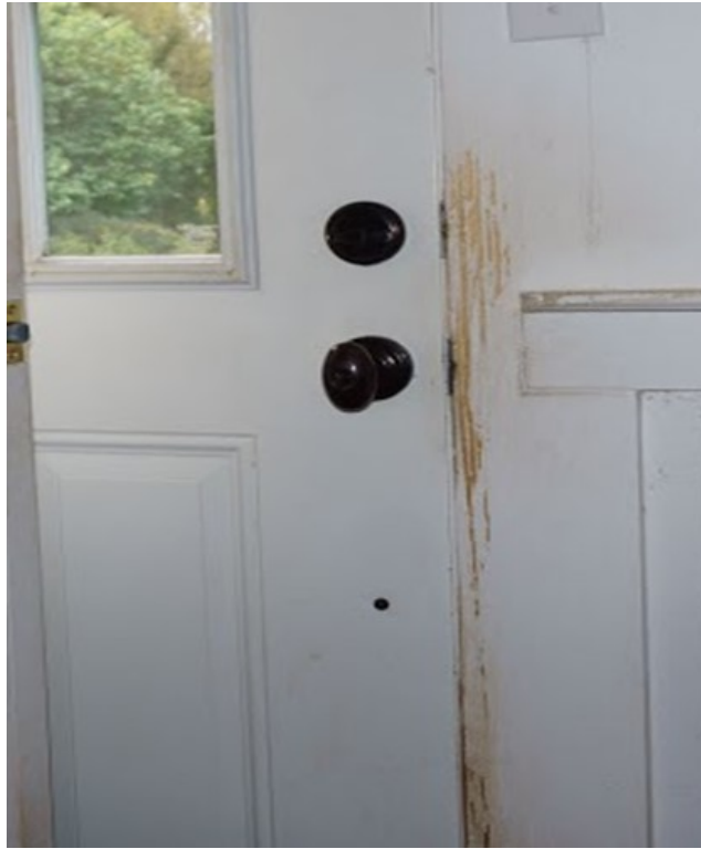
Figure 88. Missing paint along the jamb of the back door on the west wall.
