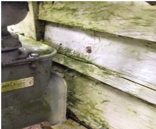
Figure 103. Mildew/rot behind gas meter on northwest end of the main house.
