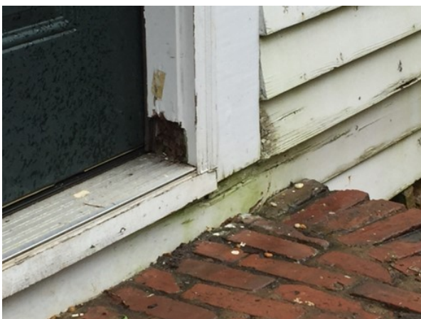
Figure 105. Wood rot on lower right corner of the back door.
