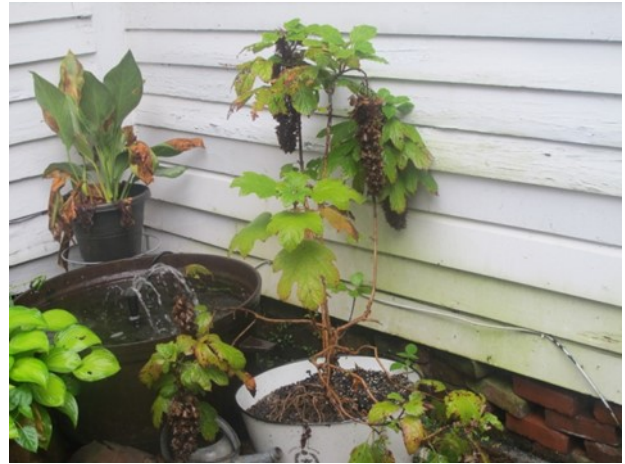
Figure 109: West Façade with vegetation too close to exterior siding.
