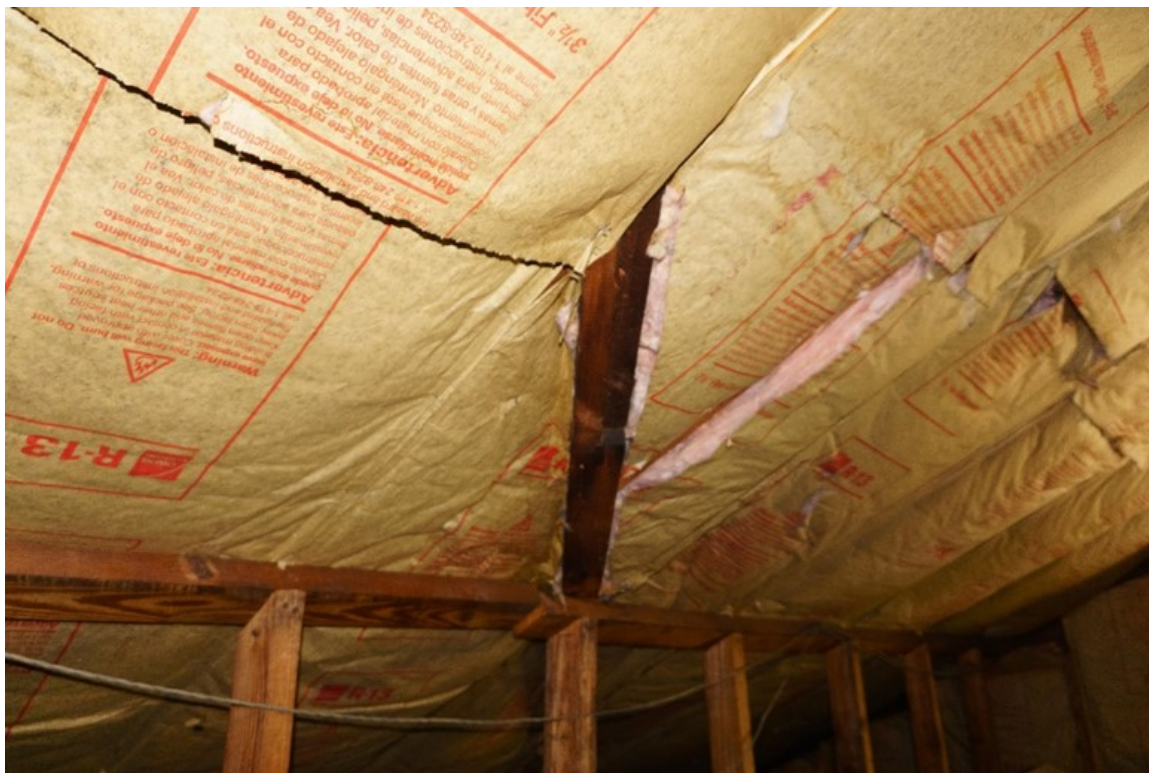
Figure 17. The historic hip beams remain in place and are visible in the attic.
