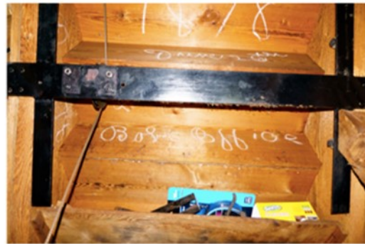
Figure 30. Graffiti in closet in Room 105.
