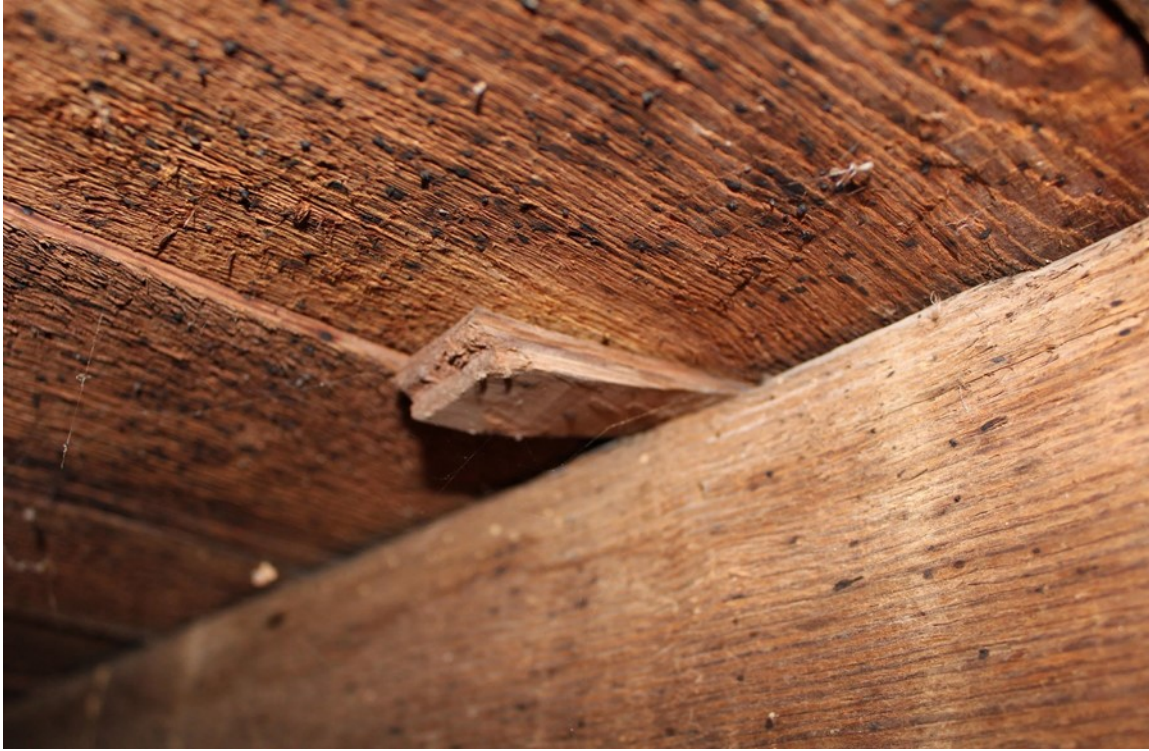
Figure 14. Joist and subfloor shimmed to fix sagging floor under Room 101
