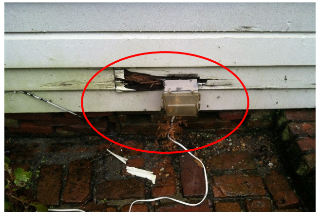
Figure 73. Rotted clapboard on west facade.
