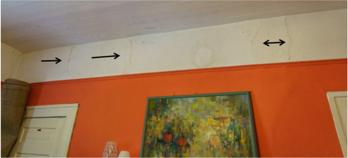
Figure 91. East wall of Room 203. Notice the cracks in the cornice.
