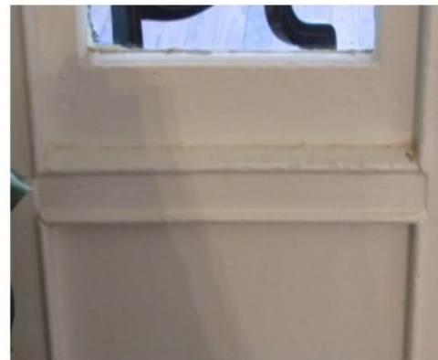
Room 105. Molding under the south sidelights of the west door. Photo by N. Gilbert, 11/14/2015
