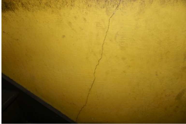
Figure 134: Attic – Vertical crack in the plaster of the stairwell leading from Room 205 into the attic.
