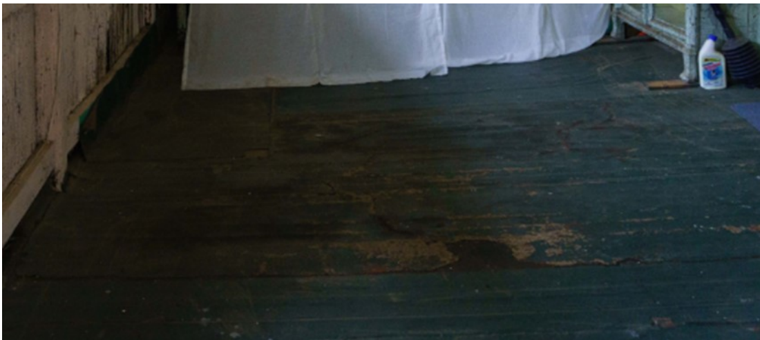
Figure 93. Damaged floor of Room 206.
