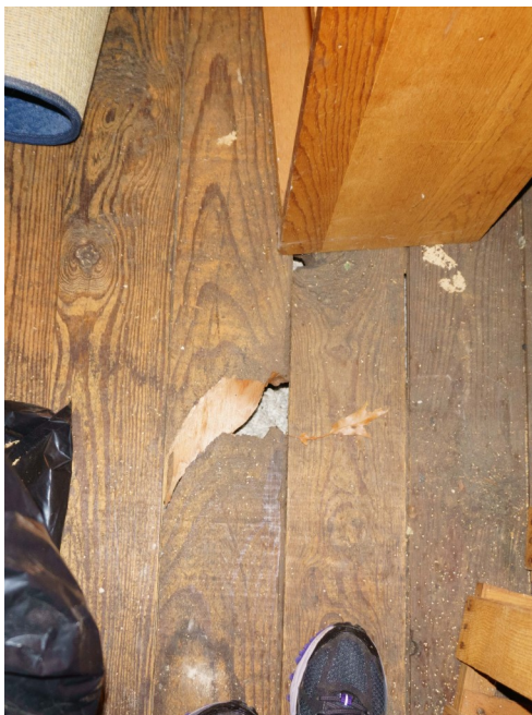
Fig 64 Attic: Hole in the wood floor.
