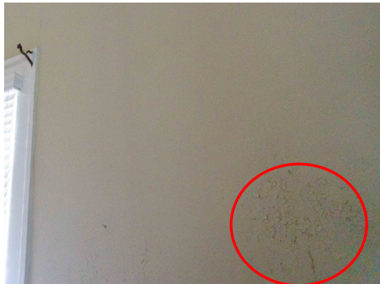
Figure 83. North wall of room 104. Notice the crazing in the lower right hand corner.
