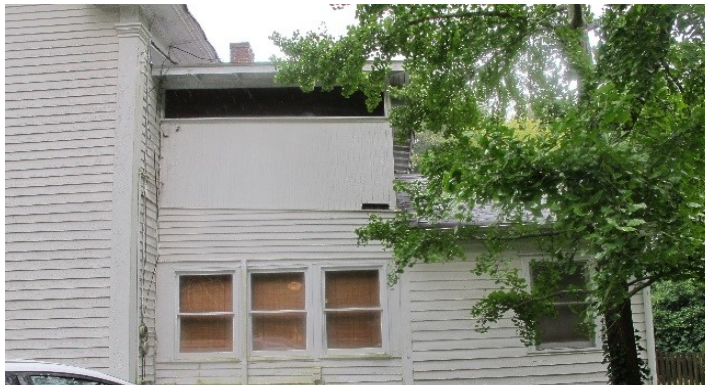
Figure 74. Vegetation too close to house and leaking gutter have formed a moisture rich "microclimate" which is causing the siding to deteriorate.
