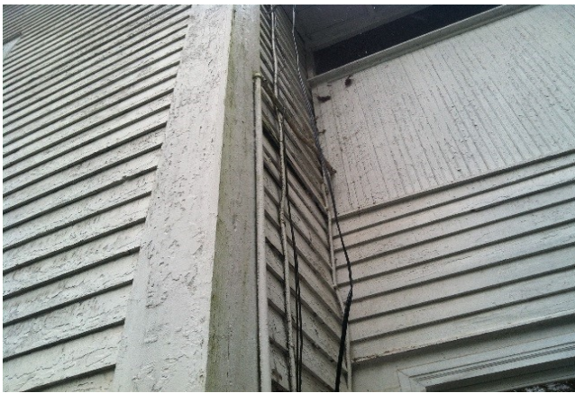
Figure 72. Paint cracking on north facade.
