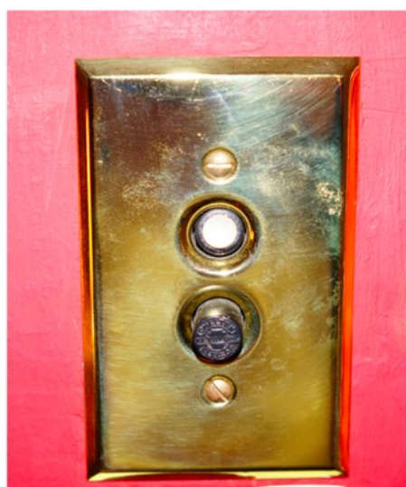
Figure 24. Two-push button light switch in Room 101.
