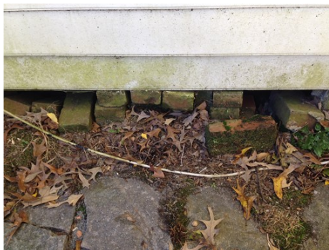
Figure 102: West façade foundation with loose and deteriorating foundation.
