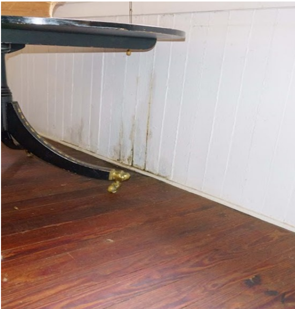
Figure 86. Rot beneath the triple windows on the west wall of Room 106.
