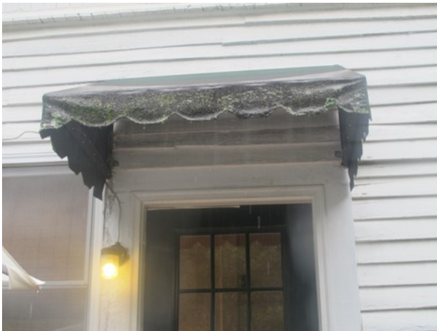
Figure 110: West Façade algae growing on awning due to excessive water.
