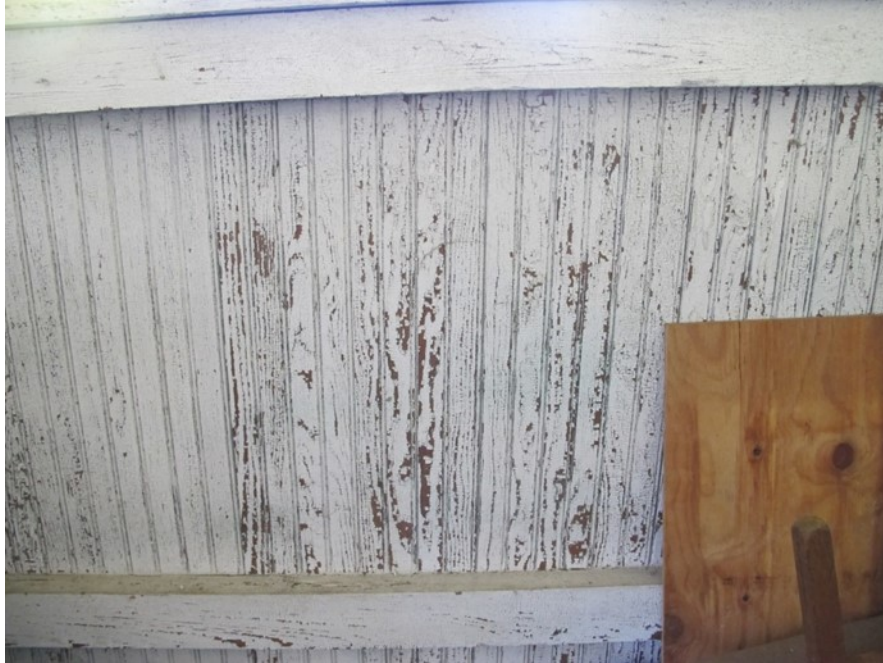
Figure 96. Alligatoring of paint on the north wall.
