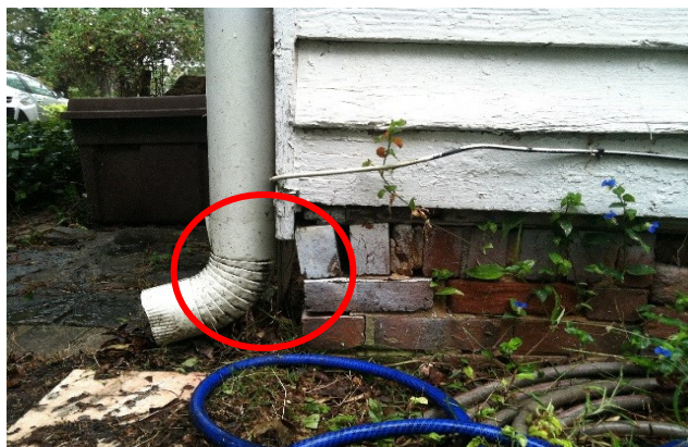
Figure 71. Foundation pier with deteriorated mortar, vegetation along foundation bricks, and gutter with no downspout extender.
