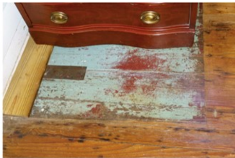
Figure 35. Room 106 ghost mark built-in northwest corner.
