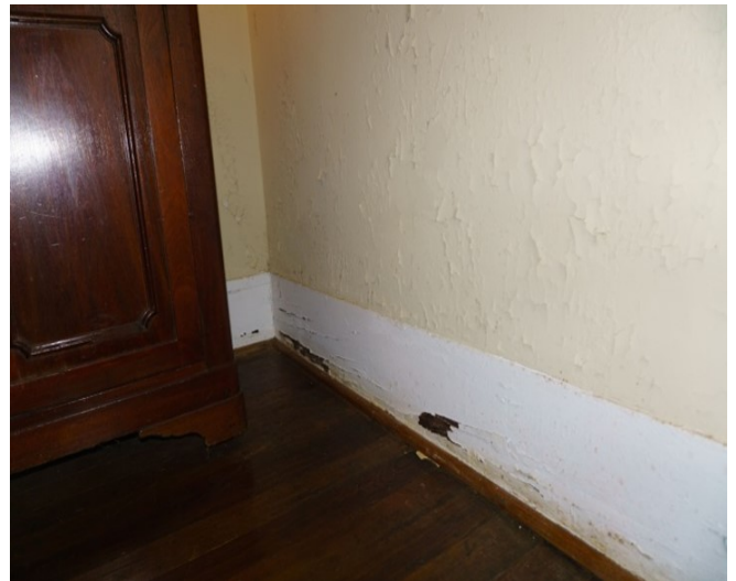
Figure 81: North wall of Room 103. Crazing above the baseboard, left of the window.
