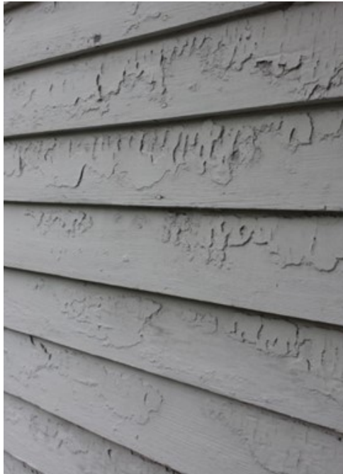
Figure 107. Alligatoring of paint on the east façade of the main house.
