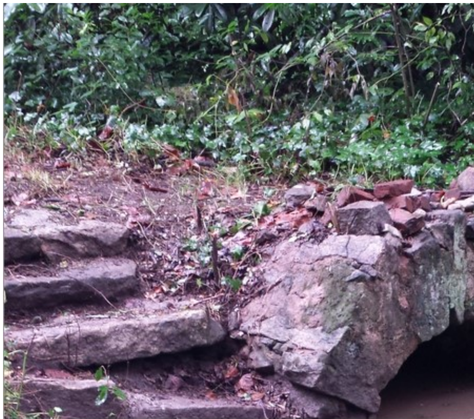
Figure 68. Vegetation grows unchecked over the masonry spring house.
