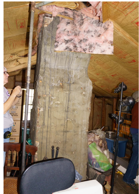
Figure 65 Attic: Chimney coated with Portland cement and brick.
