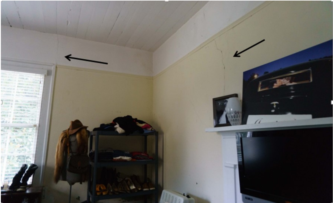
Figure 89 South and west walls of room 201. Note the cracks in the plaster.
