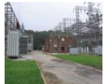
Georgia Power Substation
