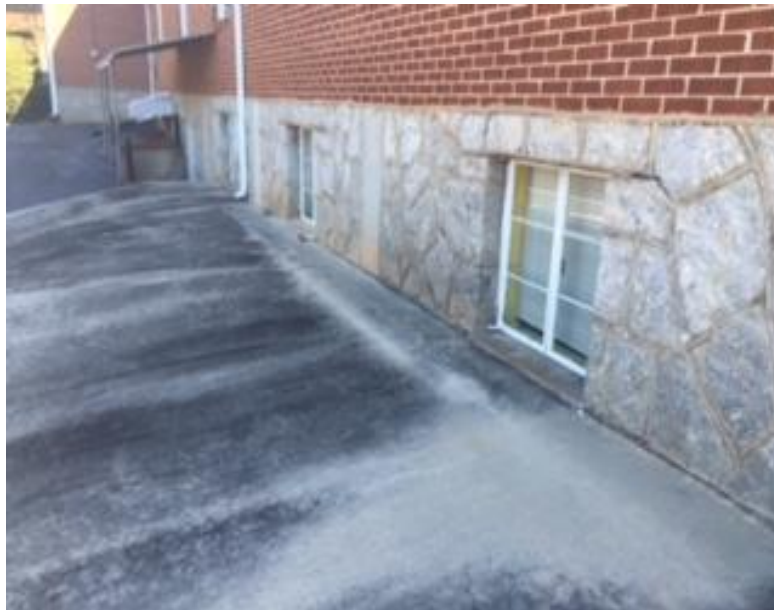
Philadelphia Baptist Church at 6910 South Goddard Road. Example of a granite foundation.
