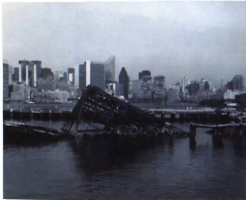
Figure 15 Current waterfront conditions found along the once thriving docks off of Brooklyn.
