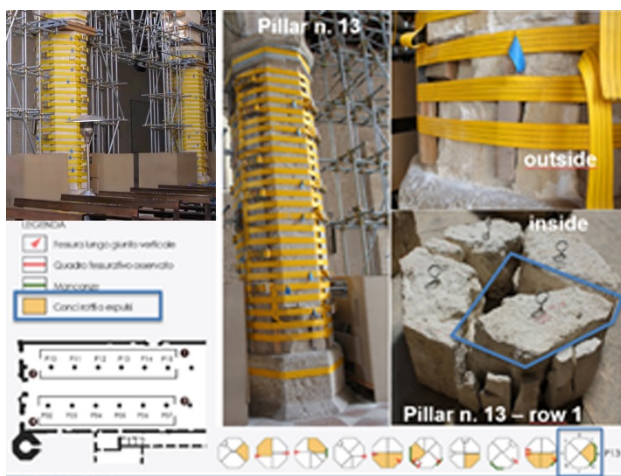
Figure 10. Pillar n. 13. A case of better ashlar stone conservation with respect to the hypothesized state of the art of the inner before disassembly and after reassembly. The external deterioration of the stone, in good condition in the inner part, is evident.
