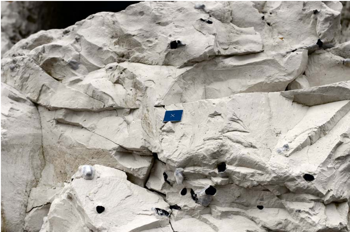
Figure 4-10. Photograph showing small scale fractures found within the Portobello chalk (0.5 m high), looking north. The nodules within the chalk are flint and chert.
