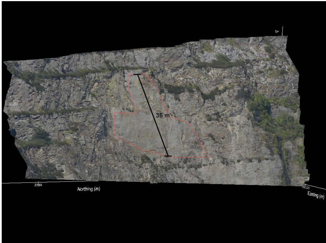
Figure 4-48. 3D image showing the 1967 failure plane (highlighted red), Delabole Quarry, Cornwall, UK. It is considered that there has been little change in the slope profile since there has been no significant failure subsequently in this regularly monitored face. The camera positions had restricted views of the lower half of the pit slope, so only the upper part, which includes the failure surface, was modelled.
