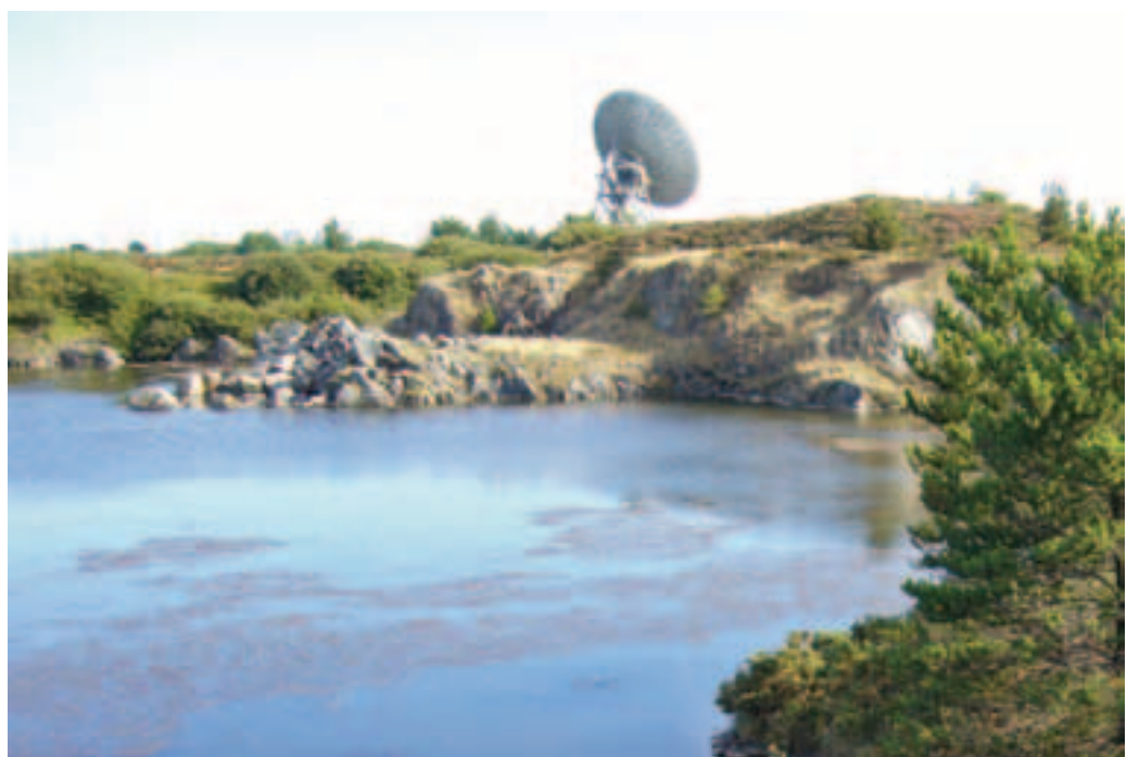
Abandoned quarry within an area designated as open access land under the Countryside and Rights of Way (CROW) Act 2000. The quarry presents hazards of unstable faces next to deep water. Countybridge Quarry, Lizard, Cornwall.
