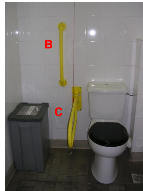
Grab rail B. Note bin incorrectly placed in transfer space. (Bichard 2005) VivaCity 2020
