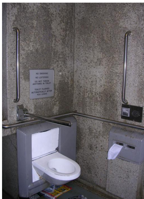
Internal fixtures and fittings of the APC do not match recommended guidelines. (Richard 2005) VivaCity 2020
