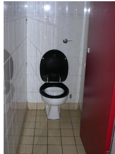
A typical standard cubicle illustrates the majority and most basic of provisions. (Bichard 2006) VivaCity 2020
