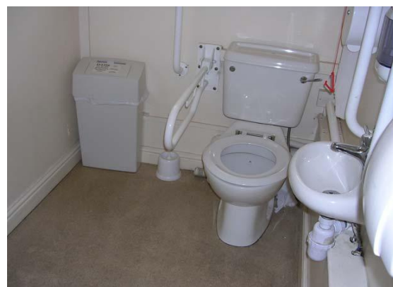
A bin placed in the transfer space of this accessible toilet. (Bichard 2005) VivaCity 2020
