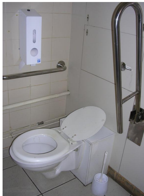
Toilets without backrests may be difficult for some users. The toilet lid may impede transfer. (Richard 2005) VivaCity 2020
