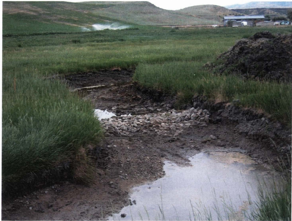
Figure 5- Section of newly constructed channel within a mesic meadow vegetation community at the Trout Creek site.
