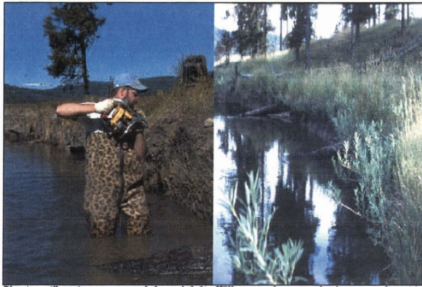
Planting willows in reconstructed channel (left). Willow growth on same bank, one year later (right).
