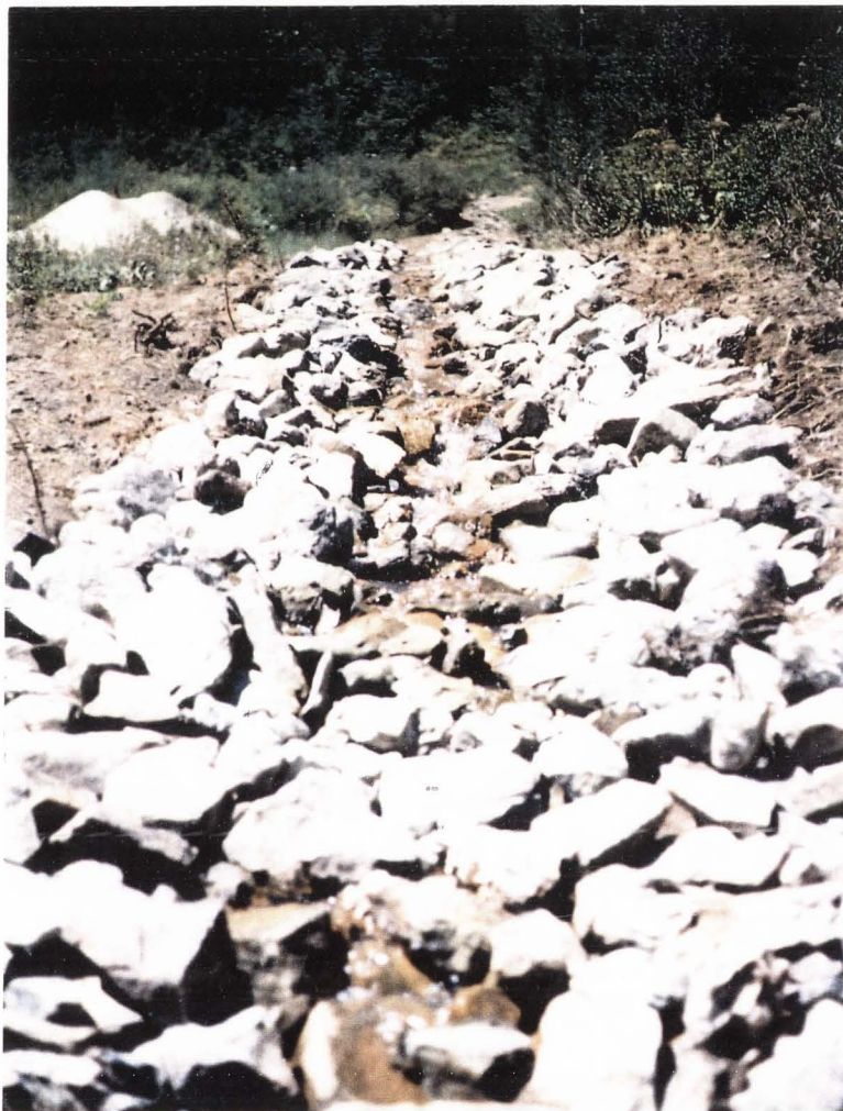
Figure 3. Diversion channel for water from the Pacific Mine portal leading into the Beaver Pond.
