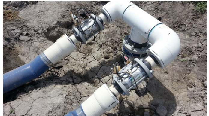
Figure 4. Water delivery line with combination pressure regulating and on-off control valve.
