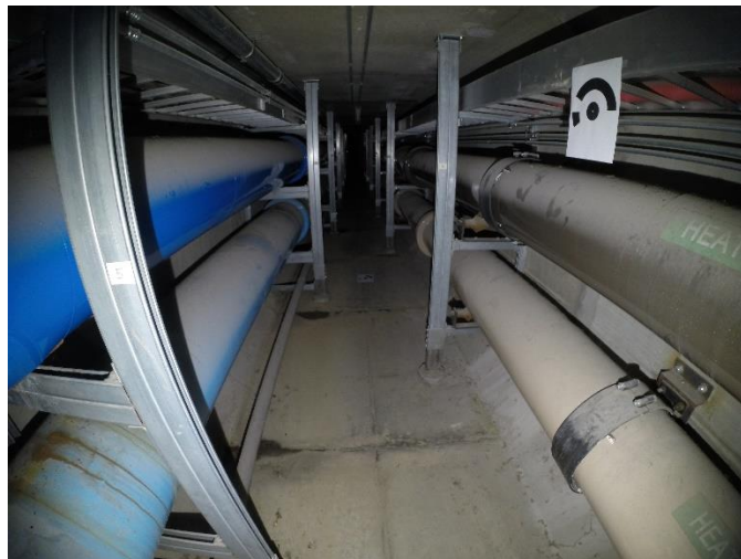
Fig 27. Severely distorted vertical support in the utility tunnel.
