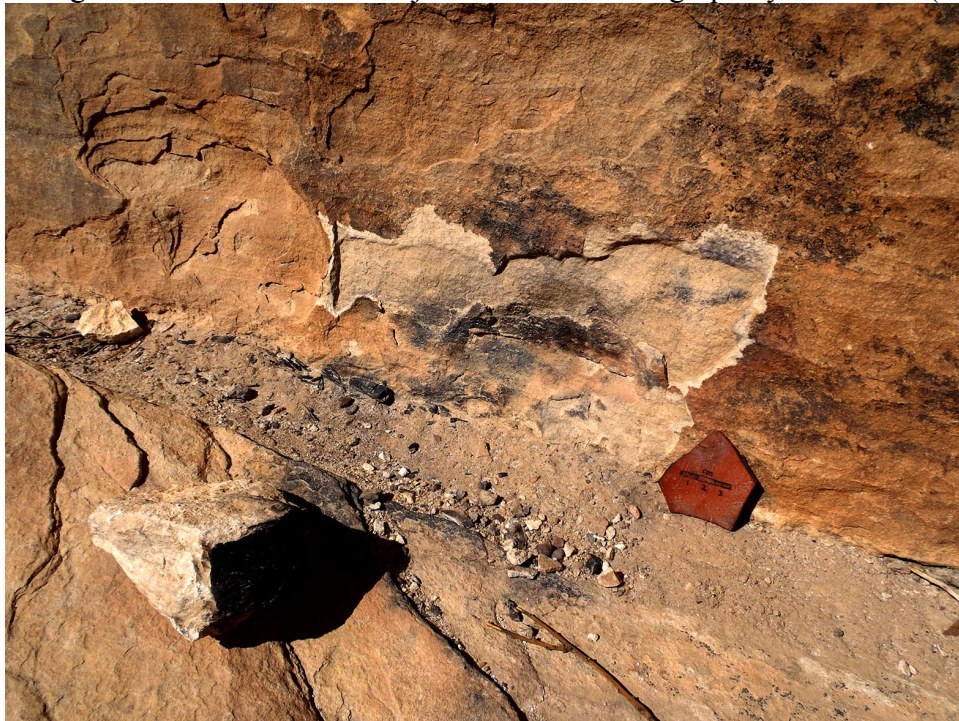
A.32: Fire damage on the eastern face of Djinn Block X. Photograph by K. Groom (2013).
