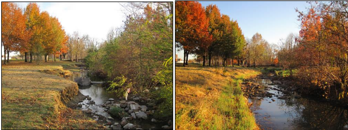
Figure 6-7: Mullins Creek before (left) and after (right) restoration efforts by the Watershed Conservation Resource Center (WCRC).
