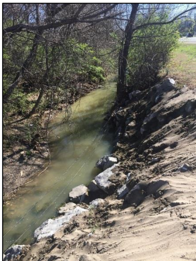
Figure 8: Existing streambank erosion at the southern end of Mullins Creek by Martin Luther King Blvd.
