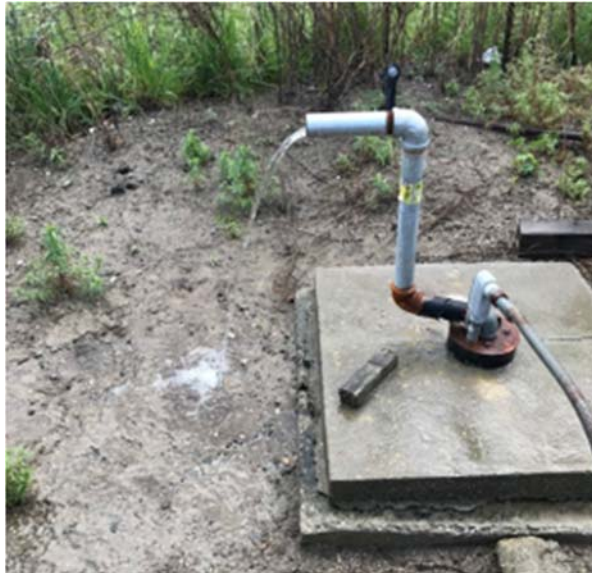
Figure 4: Contaminated well on-site at St. Francis Retreat Center.
