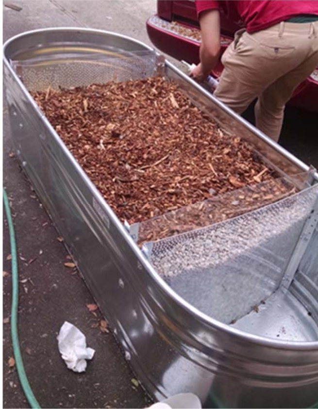
Figure 13: Beginning stages of construction. This photograph was taken after the baffle walls were installed and the wood chips and pea pebbles were added.
