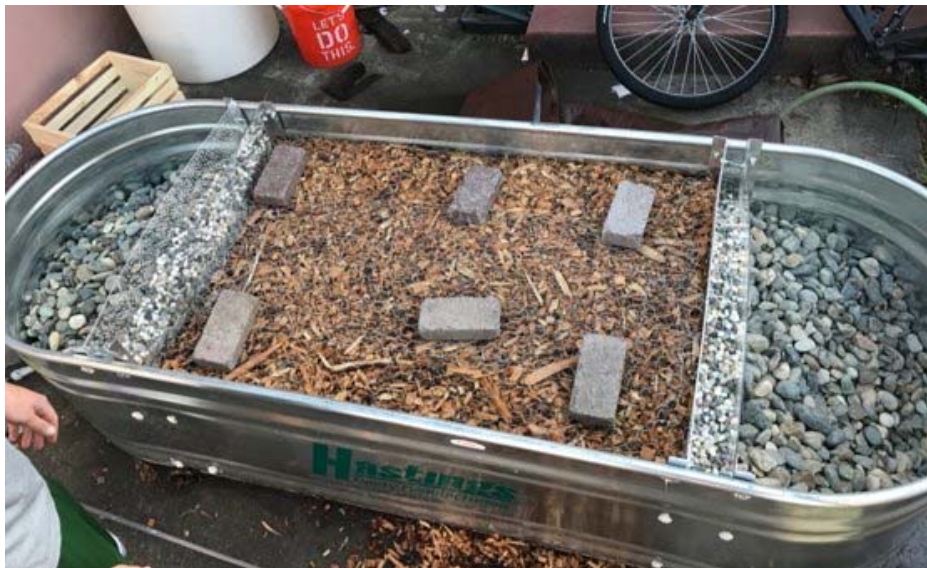
Figure 15: Late stage of construction. This photograph illustrates the bioreactor with the larger rock media and the mesh that holds the woodchips below the water surface.
