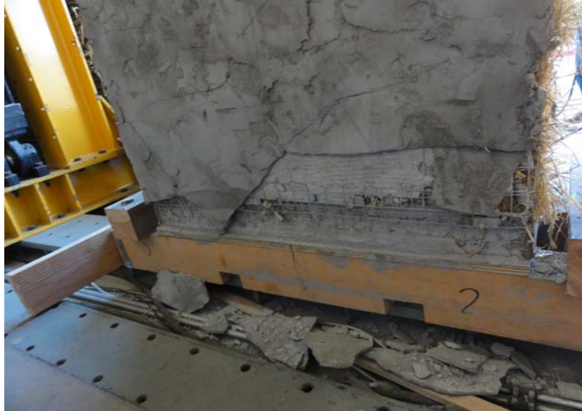
Figure 9: Outer layer of plaster delaminated from the inner layer of plaster at the base of the wall. The stapled connections of mesh to the sill plate seem to still be intact.
