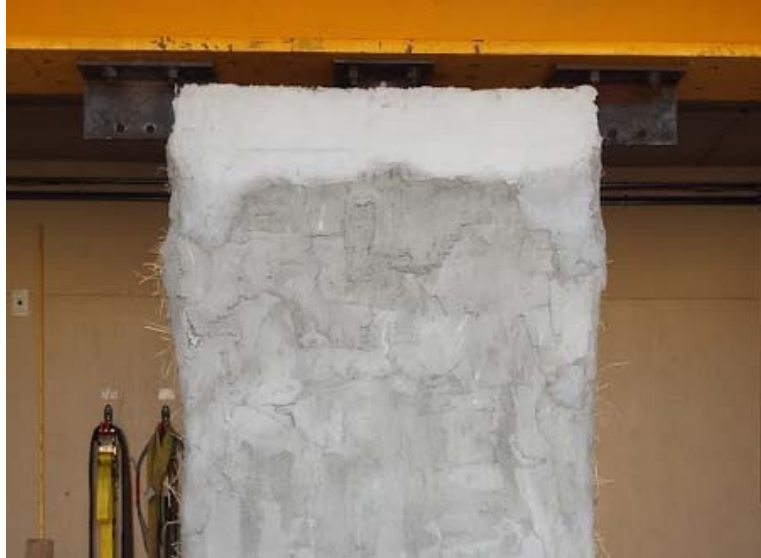
Figure 16: The new plaster can be seen here as a band of lighter plaster at the top of the wall.
