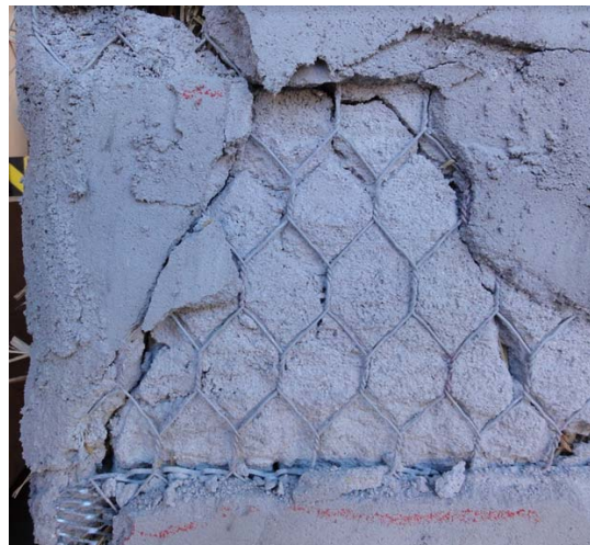
Figure 17: Taken post-lateral test. Cracks in the plaster following the “diamond” pattern of the woven mesh. Delamination is evident here where the outer layer popped off to expose the woven wire, while the inner layer remained in place.
