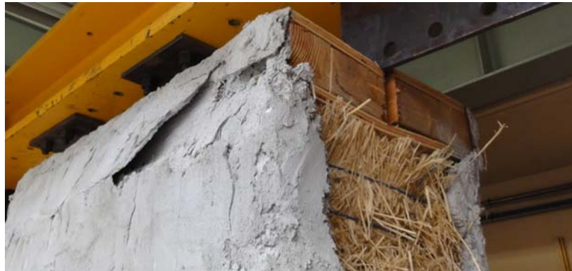
Figure 15: Crushing damage done to the top right corner of the wall prior to the lateral test.
