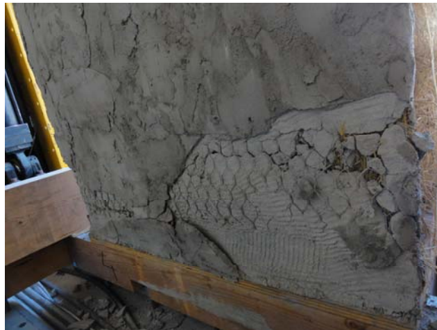
Figure 20: Backside of the Woven-18 wall, post-lateral test. Extensive delamination of the outer plaster layer has revealed the inner plaster layer. Plaster at the base remains intact and seemingly protects the stapling at the connection underneath.
