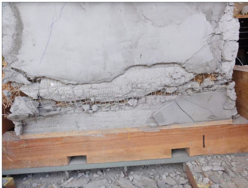
Figure 32: Damage sustained approximately 10" above the base of the Woven-14 wall after the vertical (and lateral) tests, after returning the top of the wall to its pre-test position.
