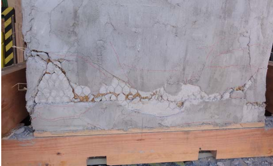
Figure 18: The damage was concentrated in a line approximately 10” above the base, due to the extra 10” band of wire mesh added to the modified workhorse connection detail, also termed the “Heckert detail.”
