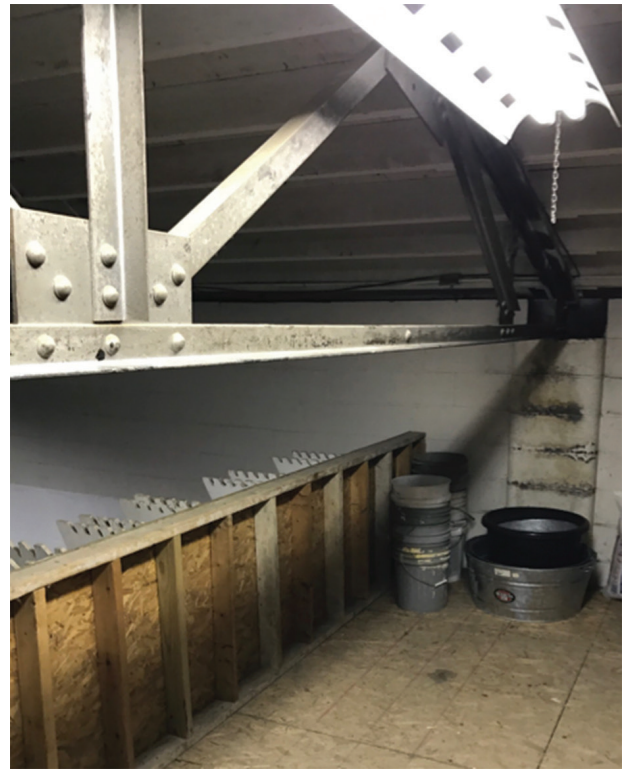
Figure 1. Example of a horizontal steel truss in the loft used to support the roof.
