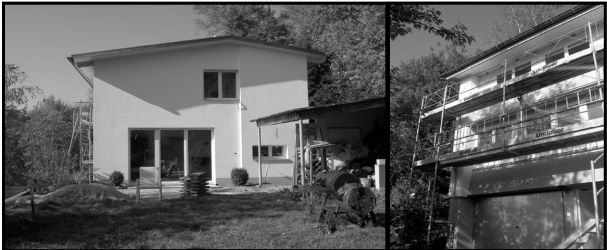
Figure 2-3: The south and the west faces of the single occupancy house during the renovation.
