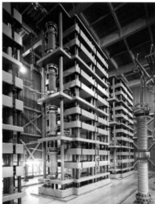
Fig. 16. Thyristor valves for the 250-kV 300-MW HVDC transmission system.
